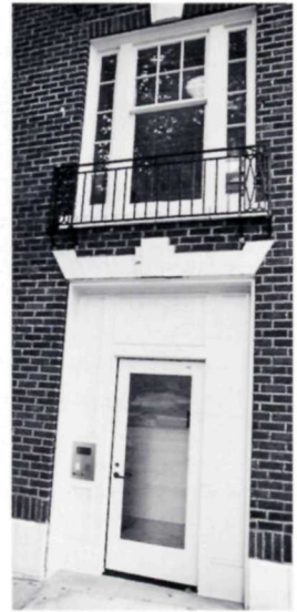
Code issues were met with creative solutions. Accessibility is provided by modifying an original window into a doorway. The balconets were retained by adding a hidden hinge allowing egress.
