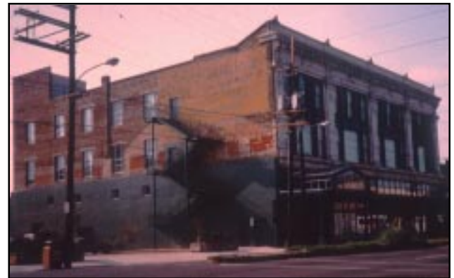
Although highly visible, because the wall is not important in defining the historic character of the building, it was possible to change the existing openings and to add several new windows to accommodate the new use.
