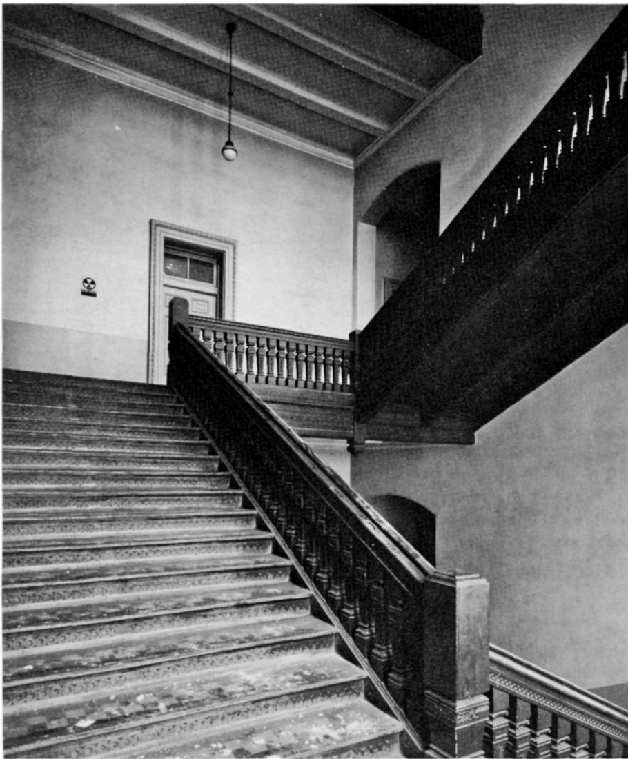
Stairway. Treads are of ceramic tile, risers and balustrades are of cast-iron. Handrail is wood.
