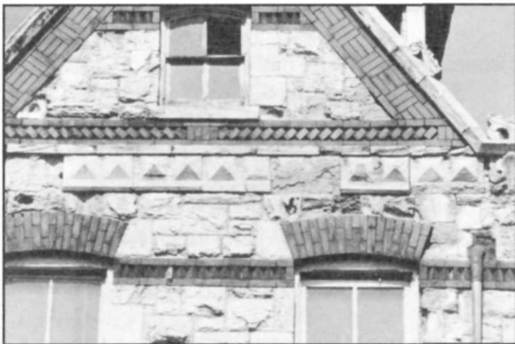
Due to extensive deterioration of green serpentine or green Maryland sandstone on the facade of this late 19th century rowhouse in Washington, DC, cast stone was used as a replacement material for the restoration. Photo: David W. Look, AIA.
