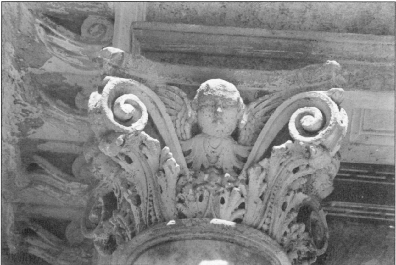
This carved limestone capital was probably painted after wind- or rain-caused erosion began to occur in an attempt to prevent further deterioration. Photo: National Park Service files.
