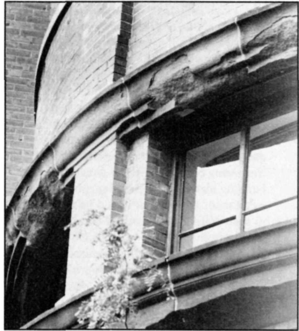
Exfoliation of brownstone lintel and sill due to the expansion and contraction of trapped moisture within the stone. Photo: National Park Service files.
