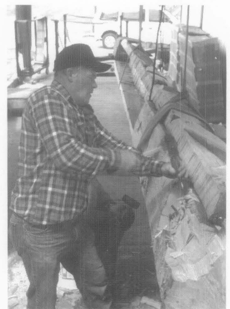
Figure 6. Three of the 7 totems had support posts. The steel bolts connecting the support posts to the totem had rusted and often needed to be chiseled out of the support post. Note the hollowed back of the totem which extended nearly the entire length while the support post extended only about half way.
