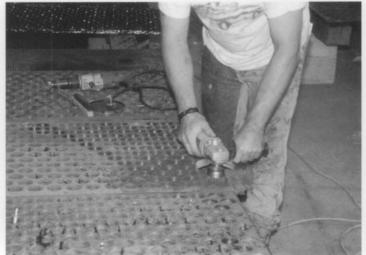
Figure 5. Workers removed any remaining corrosion, grout and other contaminants with hand chisels and power-operated wire brushes.
