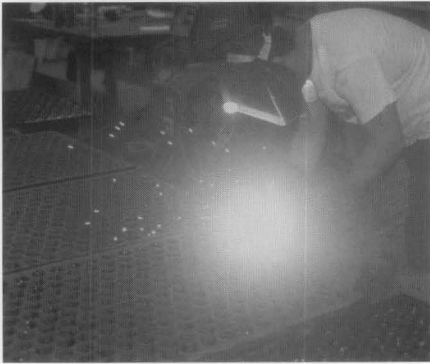
Figure 6. Cracked panels were repaired by welding in new material from a stock of salvaged panels maintained by the cast-iron contractor. The welded seams were then ground down before repainting.
