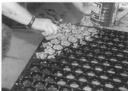
Figure 10. The grout remained water-soluble until it hardened, enabling workers to remove excess material and smooth the joint between the lens and cast-iron with a sponge.
