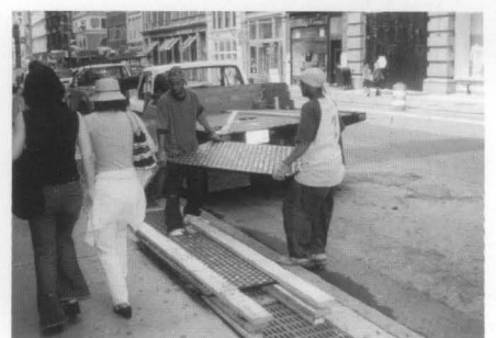
Figure 11. Just prior to installation, each panel was lifted by hand from the back of a truck and stacked on the sidewalk.
