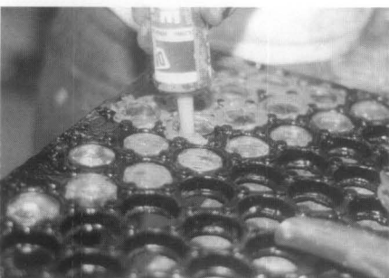
Figure 9. A caulking gun helped workers apply the waterproof epoxy grout around the lenses.
