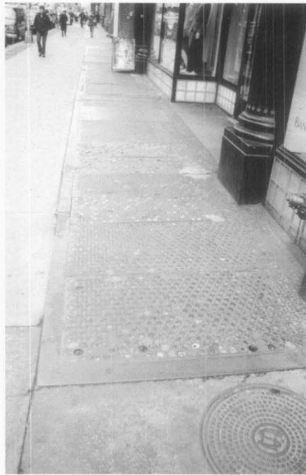
Figure 2. At the outset of the restoration project, the original cast-iron and glass vault lights in front of the building's storefront were in poor condition.
