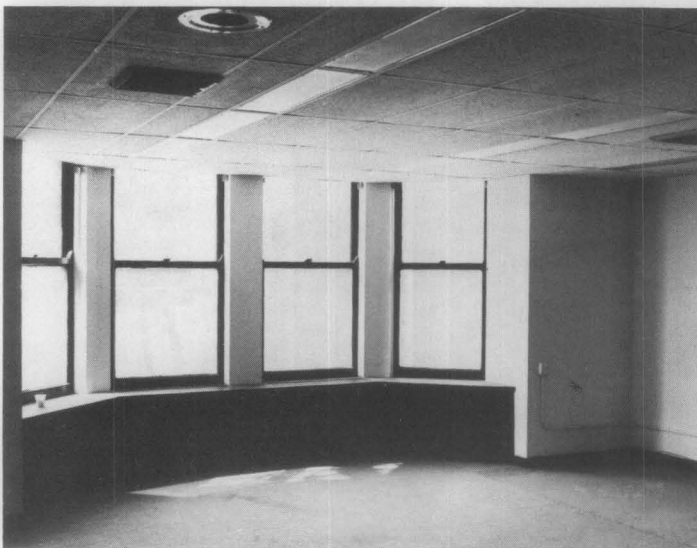
Figure 5. Typical pre-rehabilitation condition in private offices. Approximately 60 percent of all office interiors had suspended ceilings, blocked-down windows and radiator enclosures. Note inappropriate way dropped ceiling abuts windows. Photo: William S. Donnell
