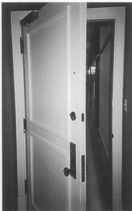
Figure 9. Fisher Building door viewed from apartment showing gypsum board infill panels, new trim and retained hardware. Photo: National Park Service File.
