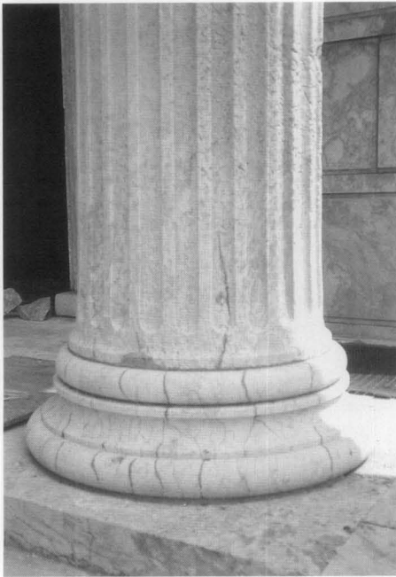
Fig. 10. The column base and plinths had extensive exterior cracks. The internal column cracks were detected by ultrasonic pulse velocity and impulse radar investigation techniques. Photo: Edmund P. Meade, P.E.
