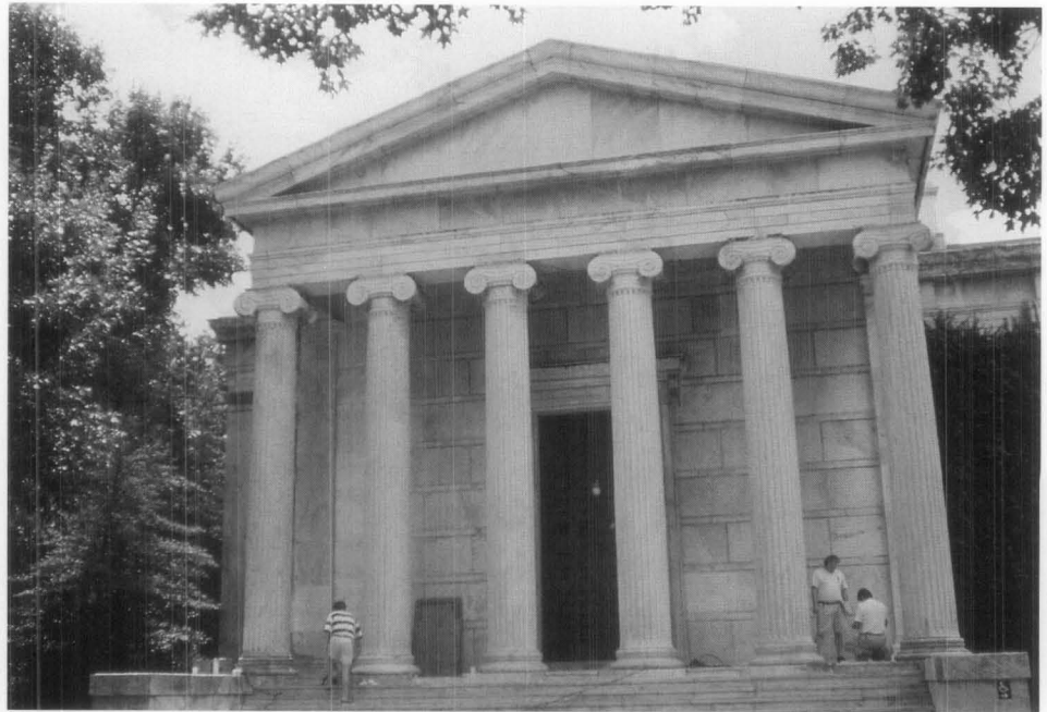
Fig 8. At Princeton University's Whig Hall, almost 100 years of weathering and a fire caused extensive damage to the masonry portico. Originally targeted for replacement, non-destructive testing techniques allowed isolated areas of damage to be evaluated and localized repairs conducted. Photo: Edmund P. Meade, P.E.
