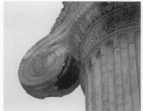
Fig. 9. The column capital volutes were cracked and spalled. Photo: Edmund P. Meade, P.E.
