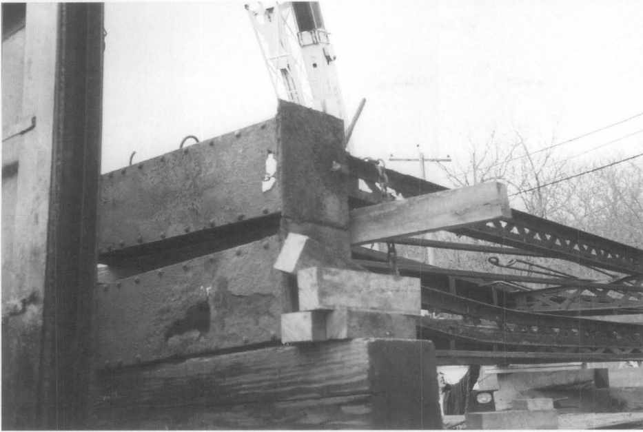
Figure 6. Although plans specified that the trusses be placed in an upright position, they were placed on the truck on their sides (left). The lower truss was damaged during the loading operation. Photo: Beta Engineering.
