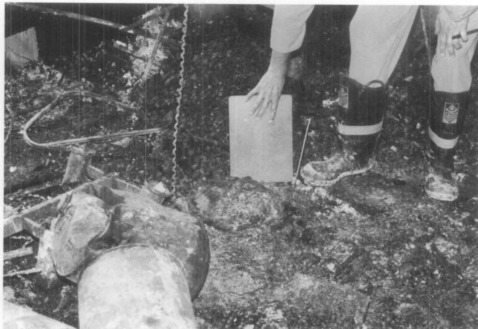
Figure 1. The spontaneous combustion of cloth rags that had been used in applying a common finishing wax caused over $1 million damage to a historic government office building in 1991. Remains of the trash can where the rags had been stored overnight is indicated by the fireman's notepad. After the cause of the fire was determined, a standard specification provision was developed for future contracts requiring the contractor to remove all material contaminated with finishing products from the site at the end of the day.
