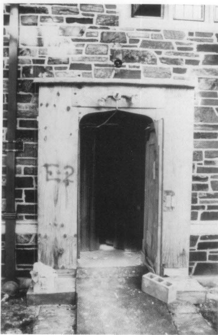
Figure 7. A contractor’s solution to protecting the limestone door surround consisted of thin foam sheeting, secured with wood nailed to the masonry. This protection was rejected as inadequate by the architect, and a full plywood enclosure constructed. In the architect’s solution, it should be noted that a temporary door is used while the original door is stored for safe keeping during construction. Photo: Ford Farewell Mills and Gatsch Architects.
