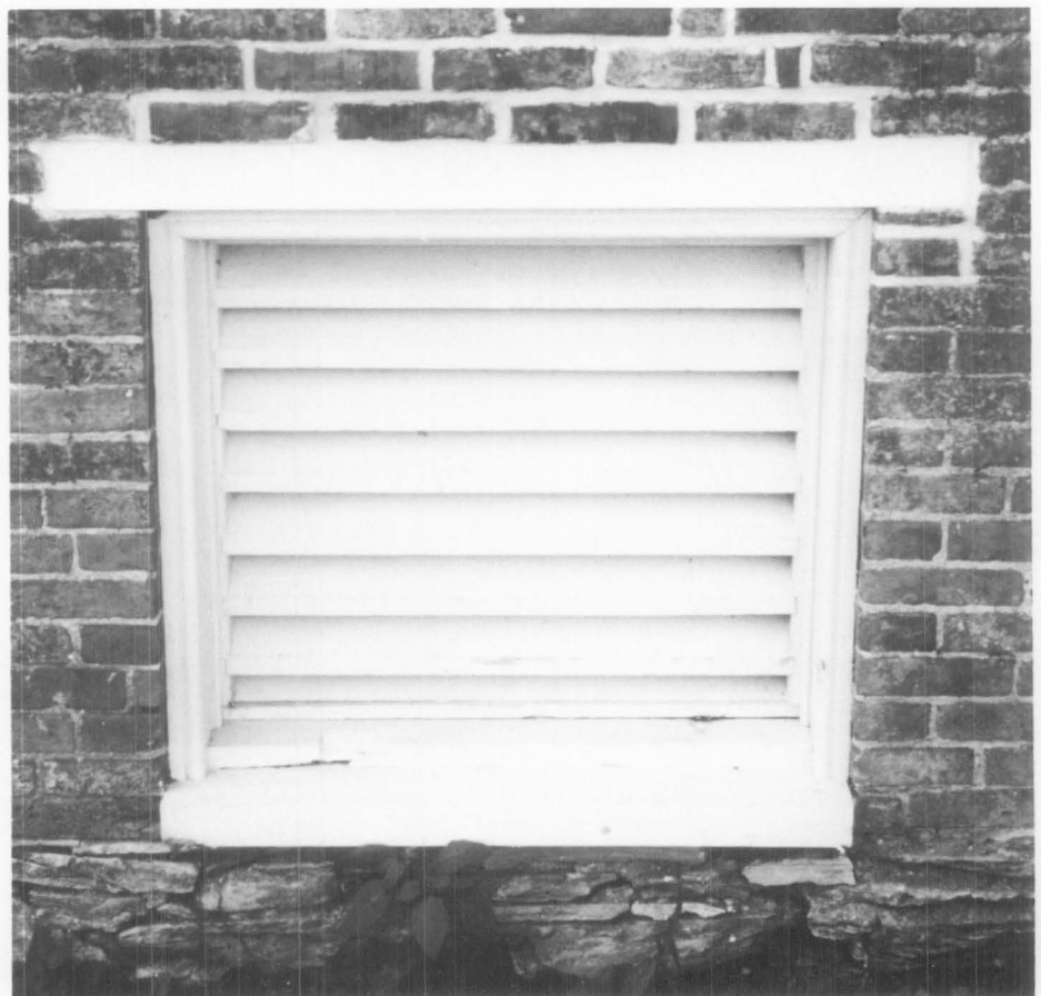
Figure 1. Full louvered vents were installed in all single-sash openings in the basement because of the more severe moisture problems present in that location. Photo: Charles Fisher
