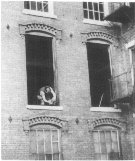
Figure 6. Work on the frames consisted largely of making dutchman repairs to the pulley stiles where required; renailling or replacing brick moldings; replacing some sills; and surface preparation. Photo: Charles Fisher
