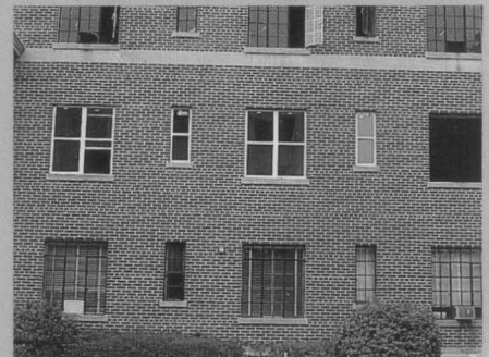
Historic steel casement windows are in the process of being replaced with new units that compromise the character of this building facade.
