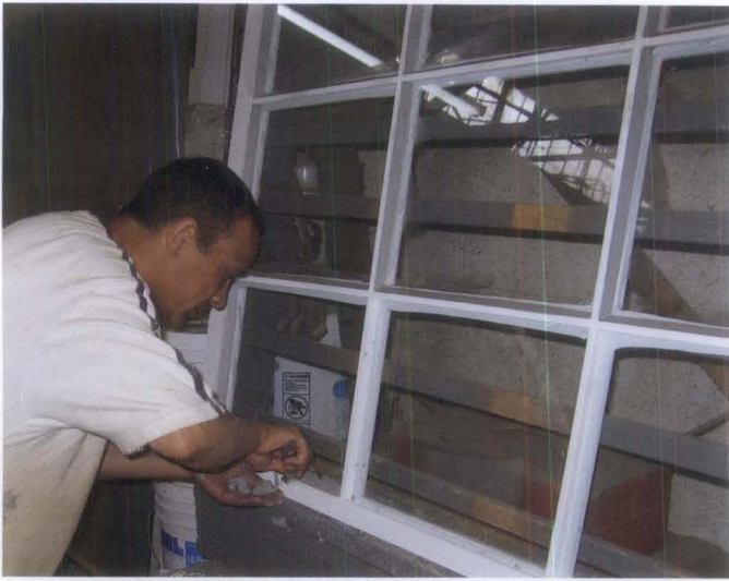
Figure 6. The outer glass was installed in the traditional manner, using exterior glazing putty. Photo: Charles Fisher.
