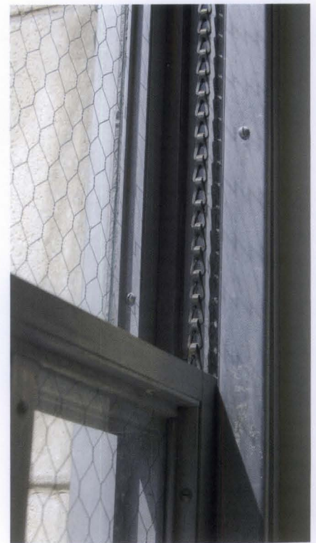
Figure 4. Early aluminum windows often mimicked wood windows in appearance and operations, even utilizing such details as parting beads, sash chains, and weights and pulleys. Photo of Folger Shakespeare Library in Washington, DC built in 1935.
