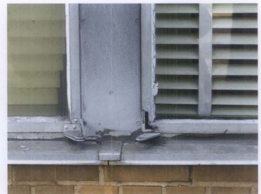
Figure 6. Deferred maintenance can result in a series of problems, such as broken hardware, cracked or missing glazing putty, and missing perimeter caulk (all shown above). All of these problems can be corrected. Note the uneven nature of the surface deposits of pollutants and grime on the mullion and sill of this window due to weathering and lack of cyclical cleaning.
