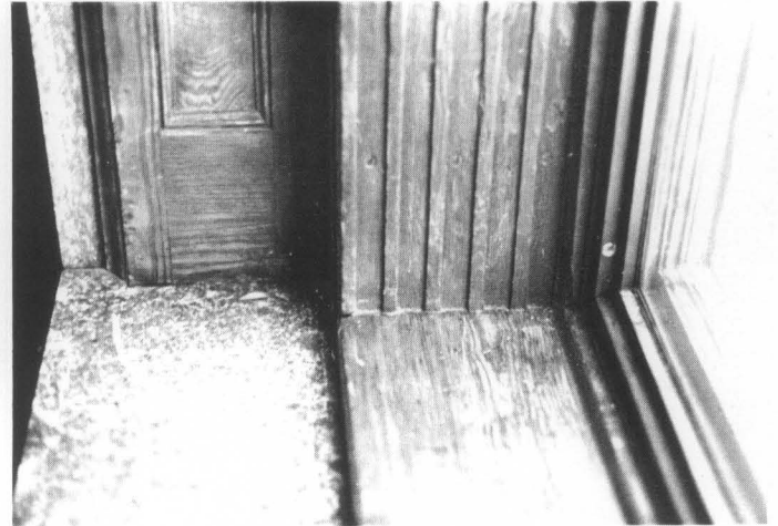
Figure 8. The decorative jamb panel on the left and the interior shutter tracks were unaffected by the installation of the interior storm window shown on the right. Photo: Charles E. Fisher
