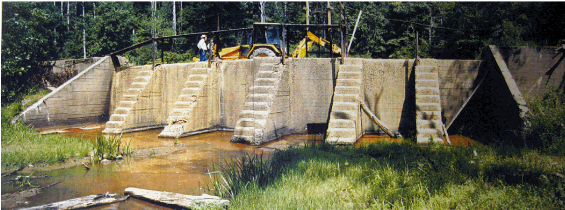
Downstream face of the dam and spillway section (1996 Examination Report PRWI archives).
