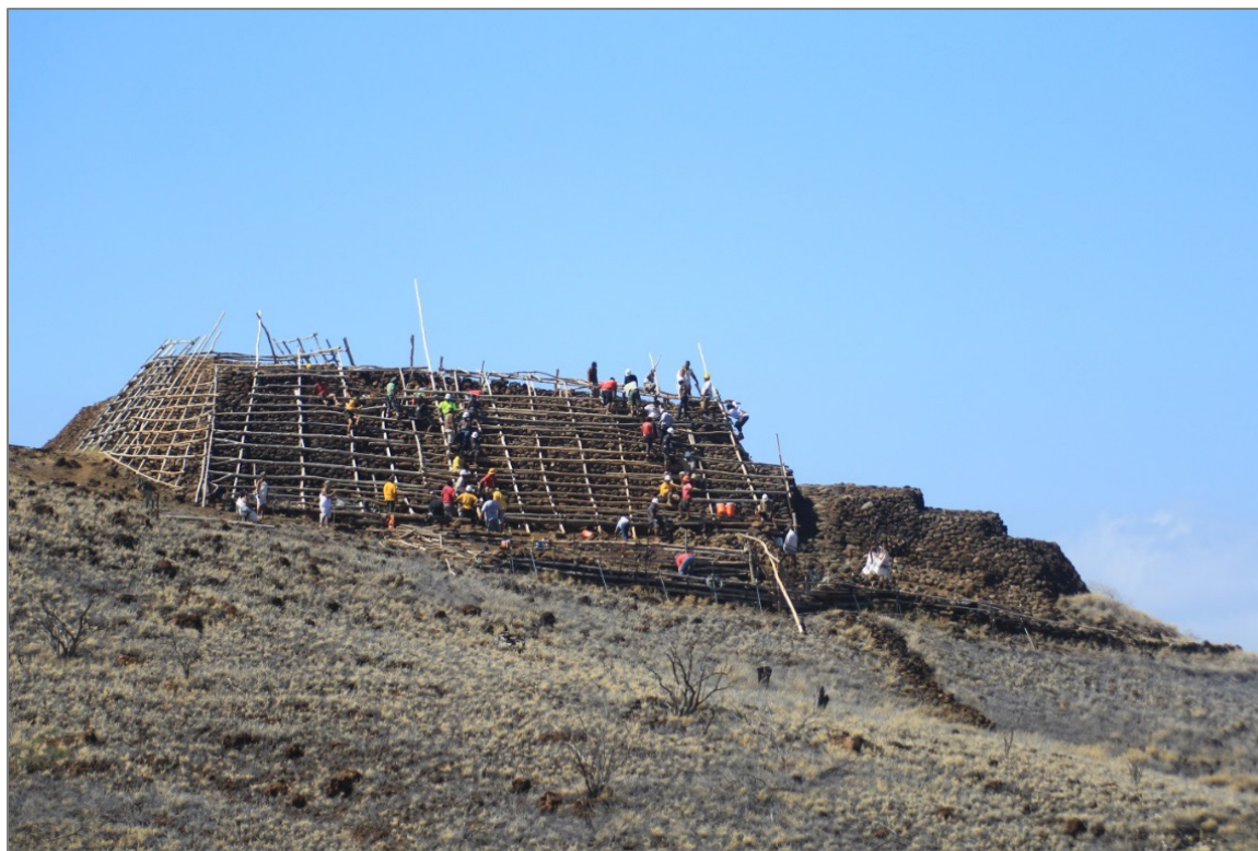
Figure 8. Earthquake repairs on north wall of Pu‘ukoholā Heiau with NPS staff and park partners (NPS photo, VIP Dave Boyle).
