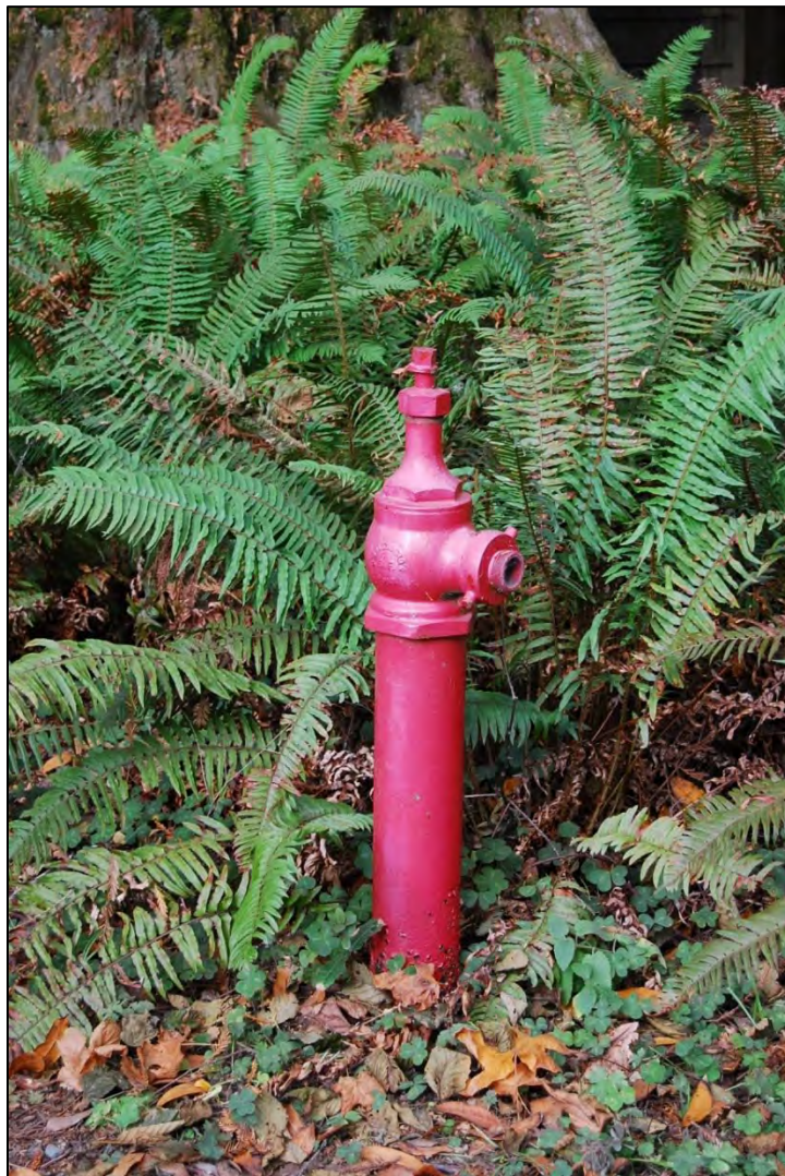
Figure 79. Small-Scale Features. Representative example of one of the fire hydrants found along Prairie Creek Road, at the Campground, and near the Garage. Additional fire hydrants are found near the Staff Residences and Boyes House.
