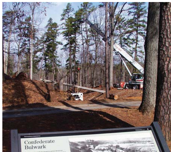
A crane lifts trees off of the earthworks of Fort Johnson, which was heavily damaged during Hurricane Isabel last fall.
