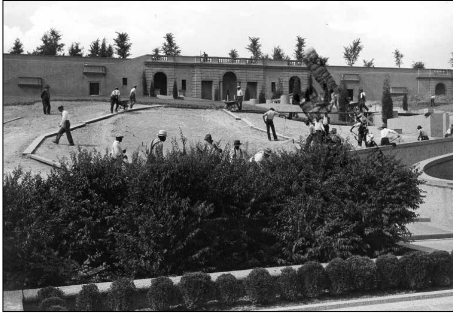
Figure 25: African American laborers starting to build the cascade portion of the Meridian Hill Park fountain (National Park Service)
