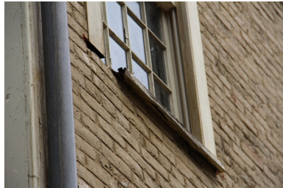
Typical deteriorated exterior projecting wood sill at masonry wall. July 2014.
