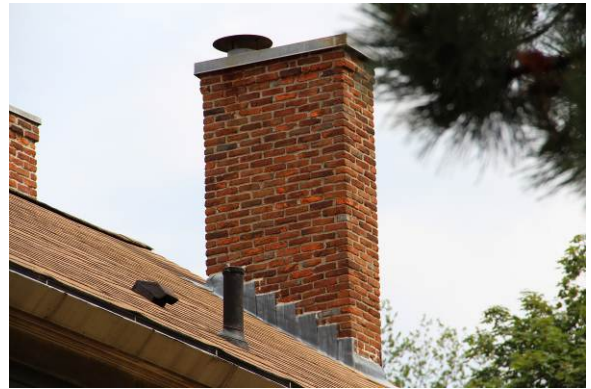
Southwest chimney (CH03) with furnace flue hood and sheet metal cap over chimney opening.
