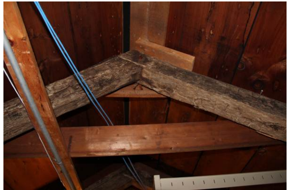
Previous supplemental bracing may not be adequate/ appropriate for historic roof frame and bearing capacity of roof system.
