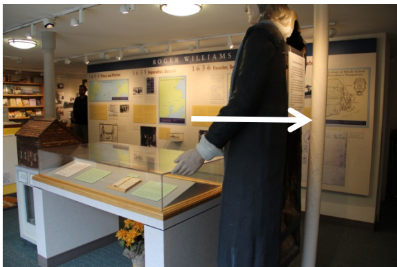
Metal column is used in lieu of original wood corner post in the visitor contact area.
