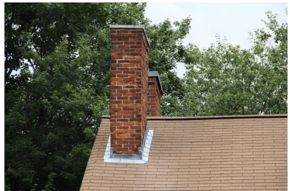
South gable chimneys seen from the east; Exposed flashing flange at base of chimneys is unusual application of base flashing.
