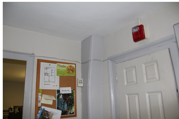
Beaded gunstock column visible on 2 nd floor is part of primary structural system (structural frame).
