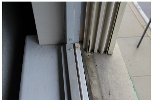
Interior / exterior view of window sills with lack of sash steps on exterior and metal interior storm window frame.
