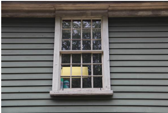
Typical deteriorated exterior window condition, July 2014.
