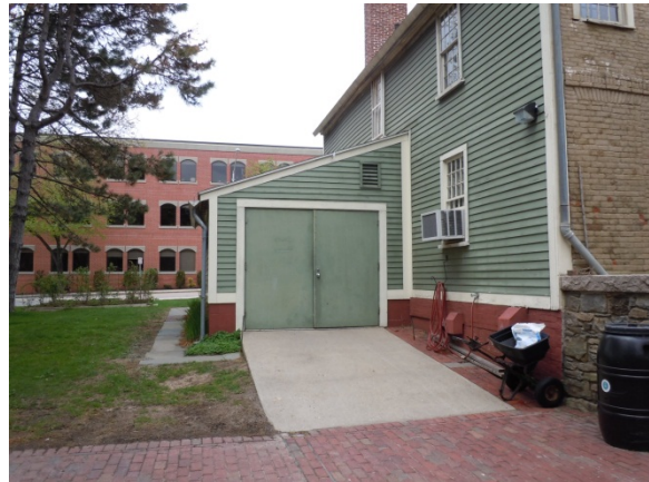
Exposed portions of foundation at west and shed elevations.
