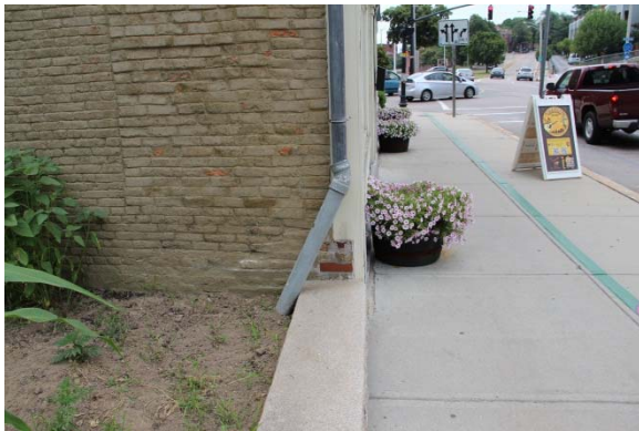
Downspout at southeast corner of building, going into an underground drain line. Connection with drainage boot pipe should be above grade level .
