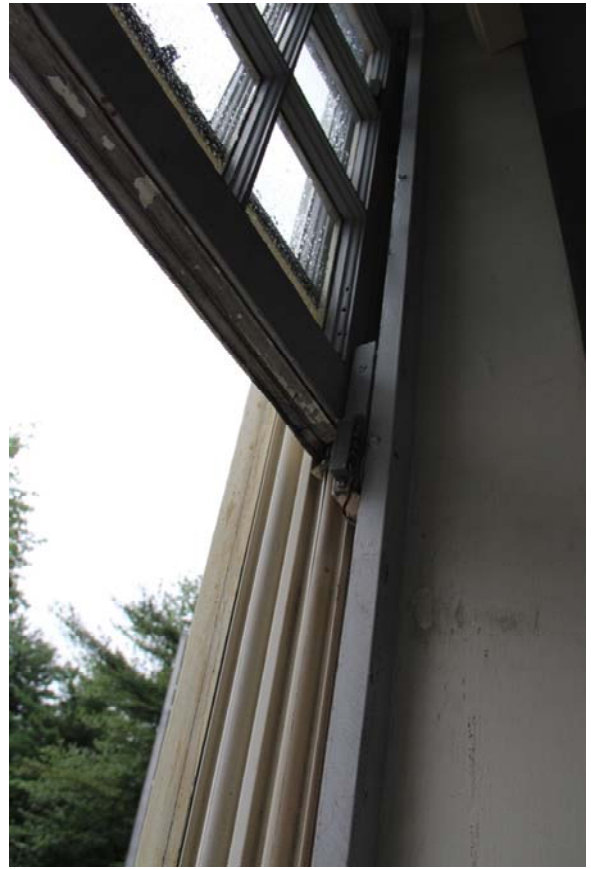
View of plastic jamb lining with sash in lifted position, note lack of weather-stripping at bottom of sash.
