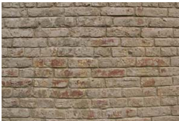
Common American bond pattern in 5 th course repeat with slightly recessed mortar joints and lime wash finish.
