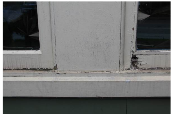
Deteriorated storefront window frame at east elevation.
