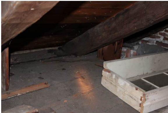
Historic rafters without supplemental supports or proper bearing at rafter plate.
