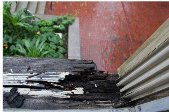
Extreme deterioration of exterior sill and jambs. July 2014
