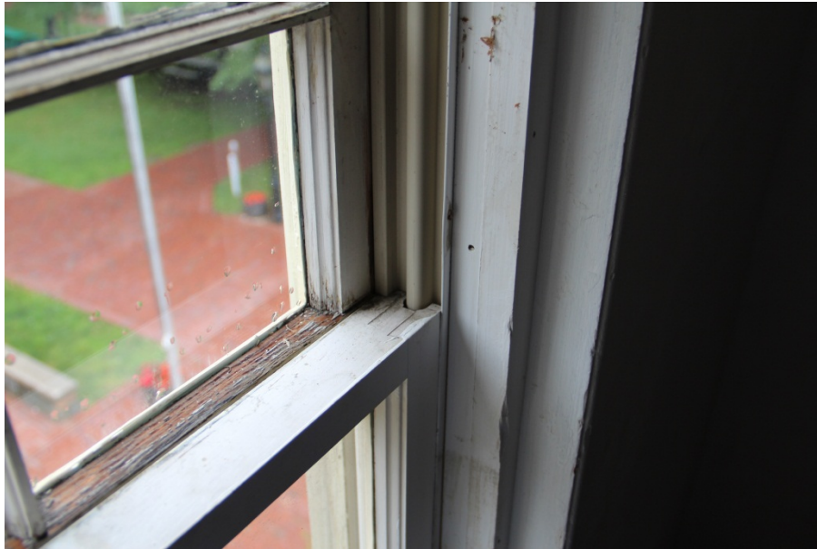
Interior upper sash frame with loss of paint and saturated wood due to water intrusion at window panes due to poor condition of exterior glazing at window.
