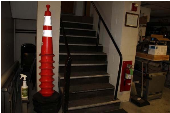
C10: Open stair between floors; also functions as main egress from basement offices.
