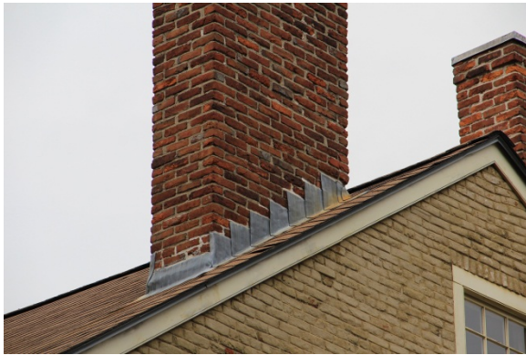
CH01 seen from the south with view of step counter-flashing and cap on chimney CH02.
