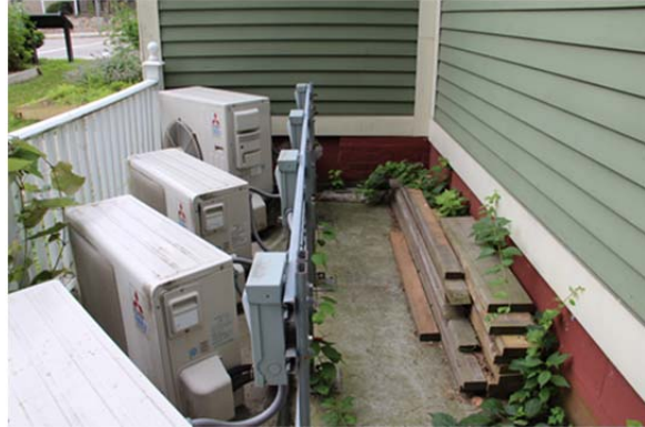
Condensing units and electrical disconnect boxes held in side yard area adjacent to primary architectural feature of the north elevation. Note storage of excess building supplies in plain view of visitors.
