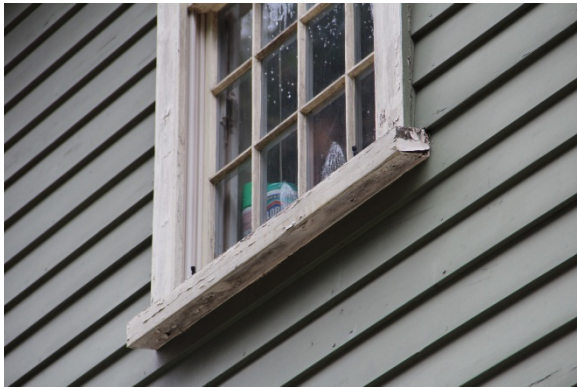
Typical deteriorated exterior projecting wood sill at clapboard siding. July 2014.
