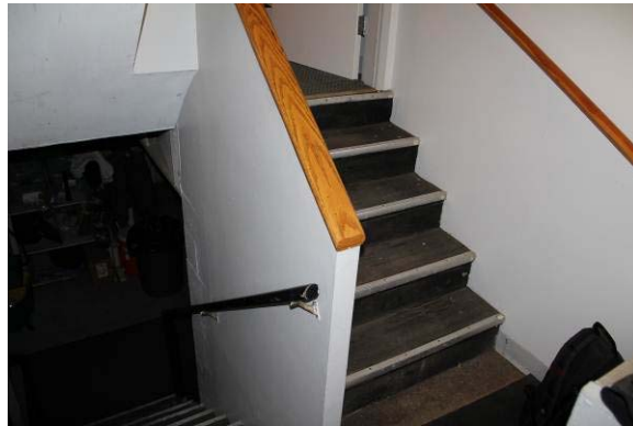
C10: Non fire rated enclosure between basement and first floor.
