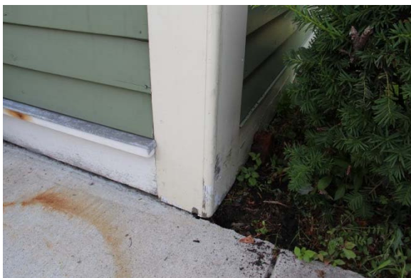
Proximity of earth and sidewalk to lower wood elements favors deterioration due to water infiltration and saturation. Flashing detail at exterior baseboard will prevent seepage into wall cavity.
