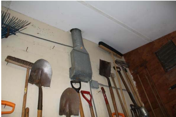
C10: Penetrations in shed ceiling negate any fire resistant separation offered by rated materials. According to NPS construction drawing it is 1/2 inch gypsum board; this assembly does not achieve a 1 hour fire resistant rating.
