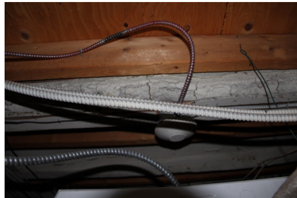
Previous generations of detectors are still in-situ above the dropped ceiling. It is unclear if these are meant to be functional or if they are operable.
