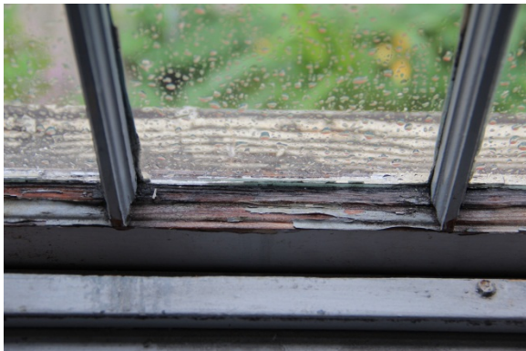
View of peeling paint on interior window sash due to similar water infiltration conditions.
