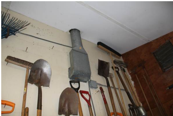
Penetrations in shed ceiling negate any fire separation offered by rated materials. According to NPS construction drawing it is 1/2 inch gypsum board; this assembly does not achieve a 1 hour fire resistant rating.
