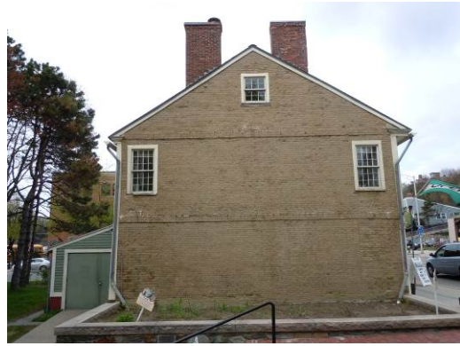
A10: Building downspouts discharge entire roof water output into plant bed adjacent to historic south brick gable. It is unclear if there is an underground drainage line or foundation waterproofing in this vulnerable area.
