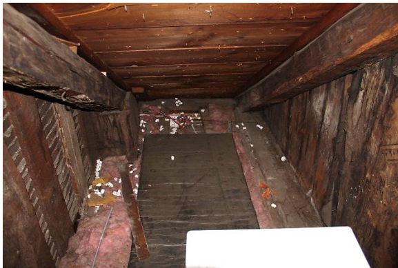
Historic rafters bear on bolster at interior post (or bearing wall) location [photo left]; rafter plate [photo right] bears on rafter plate, as is to be expected.
