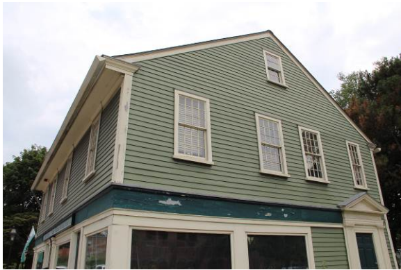
Traditional use of clapboard and wood trim are seen in 2 nd floor elevations with the various projecting ledges, corner-boards, etc., indicative of this type of layered wood framed construction.
