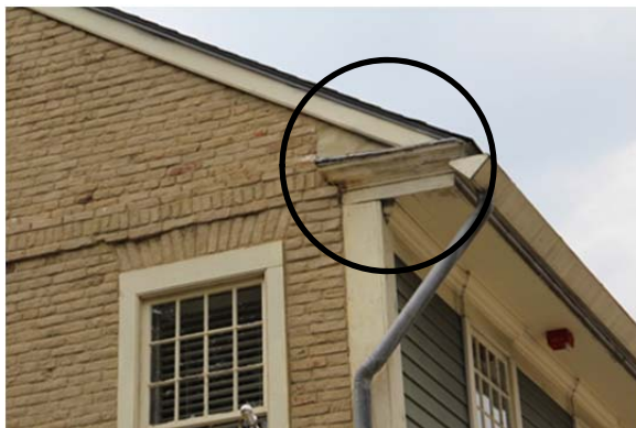
View of V-shaped hanging gutter and concealed box cornice and cornice return on building at south east corner of house. Note triangular area of infill flashing above cornice return; likely originally wood (in circle).
