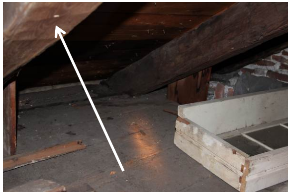
B10: Historic rafters without supplemental supports or proper bearing at rafter plate.
