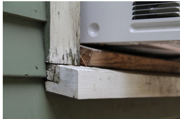
D104 – poor sill repair technique.
