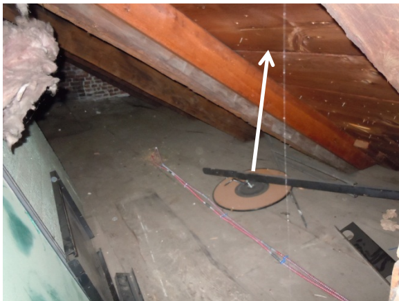
View of supplemental framing (lighter colored wood) installed along-side historic rafters. Note the roof sheathing has been replaced with modern materials.
