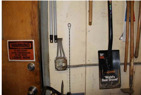
C10: Penetrations through Type X wall board (1 hour fire resistant rated material) are deficiencies in the fire rated enclosure of the maintenance shed and void the 1 hour fire resistant rating.
