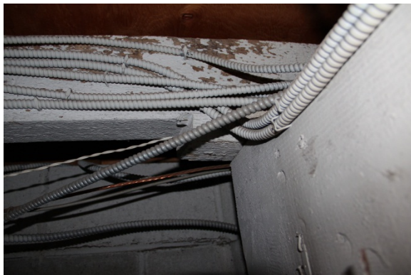
Previous installation of electrical lines and other communications systems paid no regard to labeling of wiring or attachment to National Register eligible historic framing materials.
