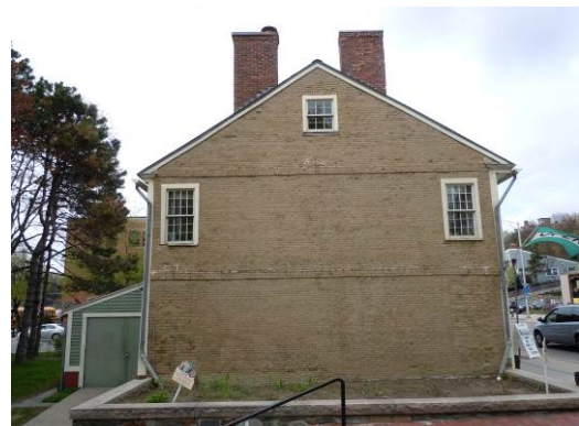
Both building downspouts discharge entire roof water output into planted bed adjacent to historic south brick gable. It is unclear if there is an underground drainage line or foundation waterproofing in this vulnerable area.
