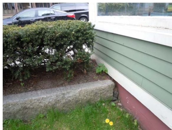
Detail lower panel under storefront showing exposed modern foundation painted red and siding in fair condition.
