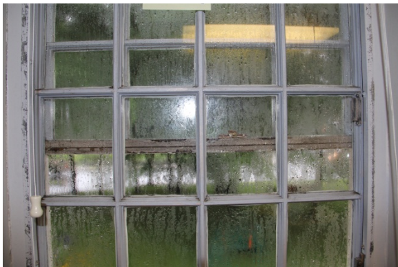
Typical interior condensation seen in July 2014.
