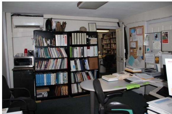
HVAC unit in-situ with exposed power and condensate lines.
