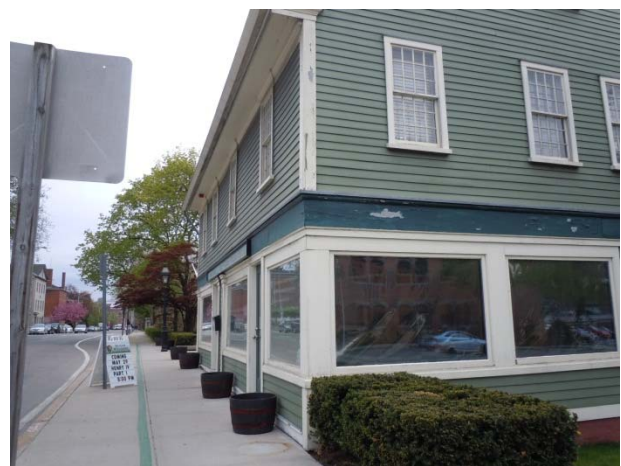
Minimal drainage along North Main Street sidewalk and building.
