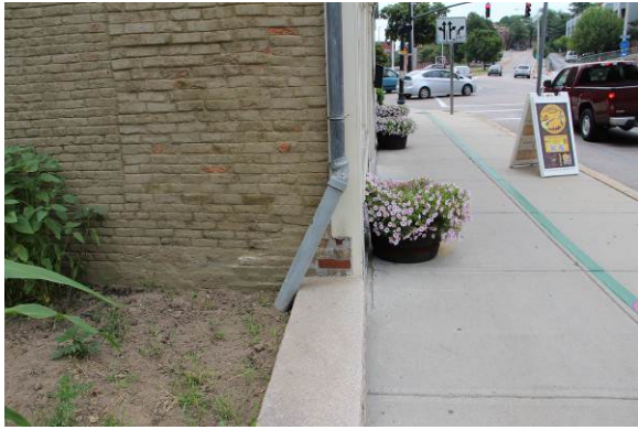
A10: Improper installation of downspout connection to underground drainage system.
