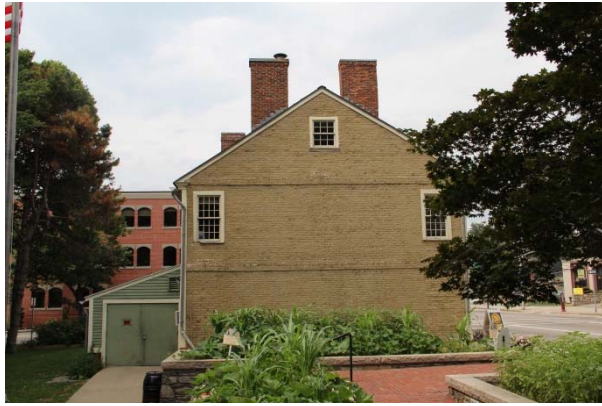
Vegetation in planter box at base of south gable wall of building. It is not known if the below grade sections of this wall have been waterproofed.
