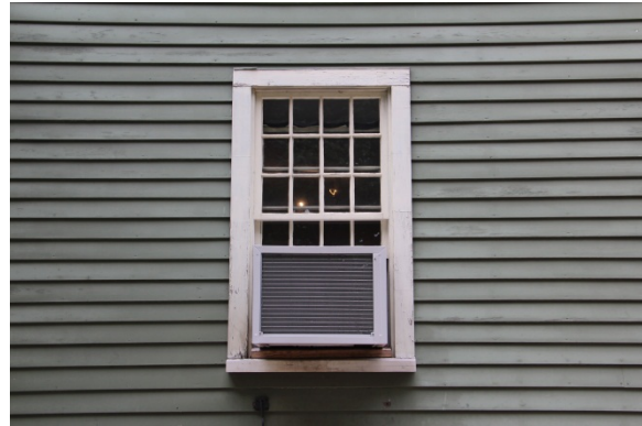
W104: supplemental air-conditioner is propped into window frame using lumber shims on exterior; window exhibits signs of advanced deterioration.
