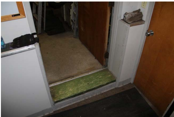
D104 threshold between house and maintenance shed; door is delaminating at the base and weather-stripping is rabbeted into door; this likely voids any fire rating the door may have had from the factory. No UL rating was found on the door.
