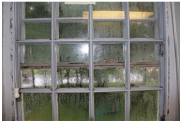
D30/ B20: Condensation on interior of window glass in summer indicates high interior humidity levels and use of uninsulated glass in windows.
