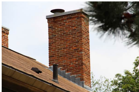
B10: Southwest chimney (CH03) with furnace flue hood and sheet metal cap over chimney opening.
