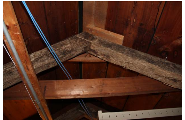
View of roof rafters pinned at ridge with replacement roof sheathing and supplemental bracing to support roof frame.
