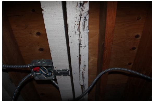
Casual observation reveals a number of electrical code violations and the concealed wiring above the dropped ceiling of the basement work areas.
