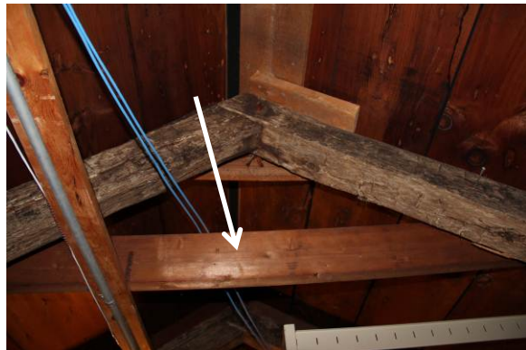
B10: Previous supplemental bracing may not be adequate/ appropriate for historic roof frame and bearing capacity of roof system.
