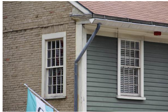
South elevation window with jack-arched lintel over wood header and projecting wood sill and east elevation with integrated lintel and projecting wood sill.
