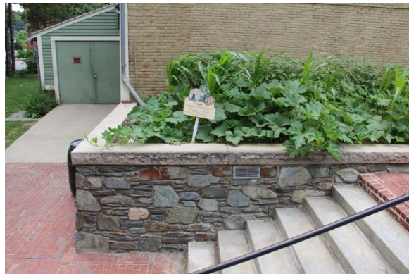
Similar condition at southwest corner of building.
