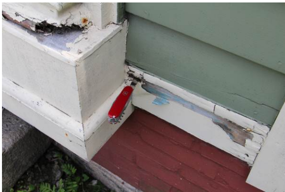
Deteriorated exterior building features at north elevation door.
