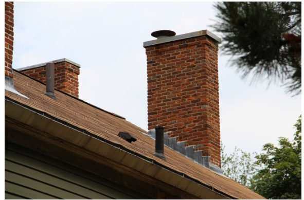
CH01 seen from the northwest; all roof penetrations are on the west side of the roof leaving a clean appearance for the street elevation (east). Chimney caps are seen on both south gable chimneys in this view.
