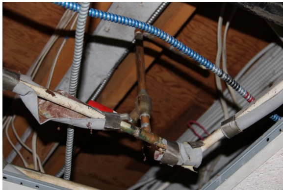
Plumbing, electrical, communications and alarm system lines all held within interstitial space above basement dropped ceiling.
