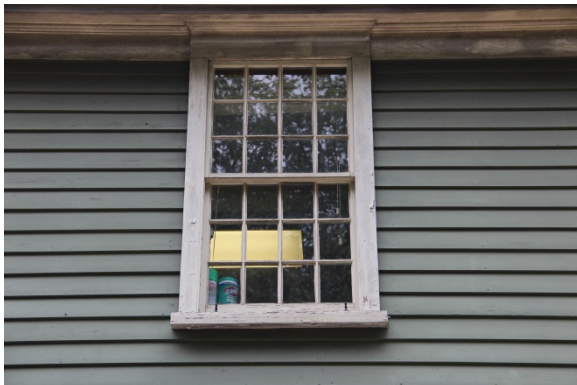
Exterior window frame with mildew, dirt and failing paint system.
