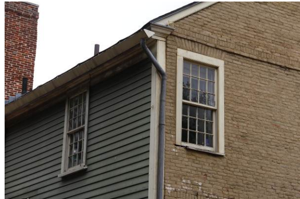
Accelerated deterioration of exterior window components, July 2014.
