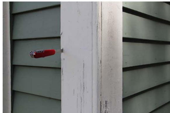
Deteriorated corner boards at northwest corner.
