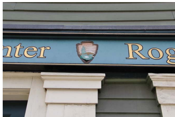
NPS park quarter-boards are faded and decals are peeling.
