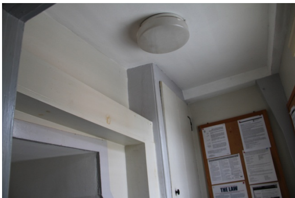
Beaded gunstock corner post and beaded floor plate beams are visible in the north entrance vestibule area (R106).
