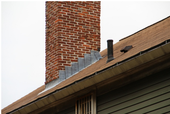
CH03 seen from the southwest with exposed step flashing; plumbing vent stack and bathroom exhaust hood seen in foreground.
