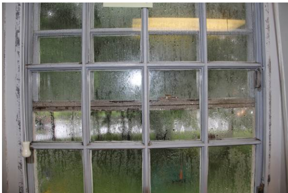
Typical non-historic replica interior window condition with interior storm window frame.
