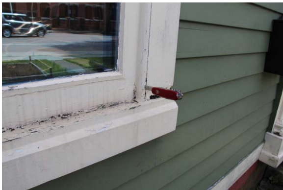
Deteriorated window trim at north elevation.
