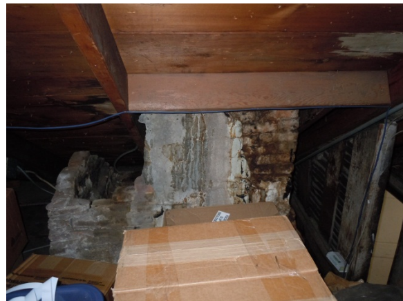
Area around chimney CH03 which has been reframed as part of a renovation project. Plywood has been used as the roof sheathing and substrate for the exterior three-tab shingle roof.
