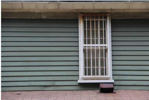
W208: exterior security grate is rusted and requires detachment from building to further inspect window sill and frame.
