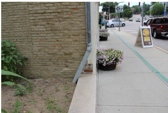
Improper installation of downspout connection to underground drainage system (may be a temporary repair).
