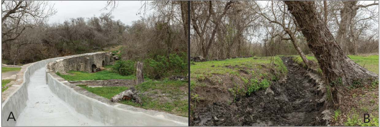
Figure 15. Views of the Espada Aqueduct. A) A view across the recently cleaned Espada Aqueduct from its top. Typically, water flows through the aqueduct channel over Piedras Creek. This channel requires occasional cleaning due to sediment accumulation. B) View of the acequia that leads into the Espada Aqueduct. This acequia was recently excavated to deepen the channel and allow for an easier flow of water into the aqueduct. Slumping does occur along the banks of this acequia. Both photos taken by Matthew Harrington (Colorado State University).
