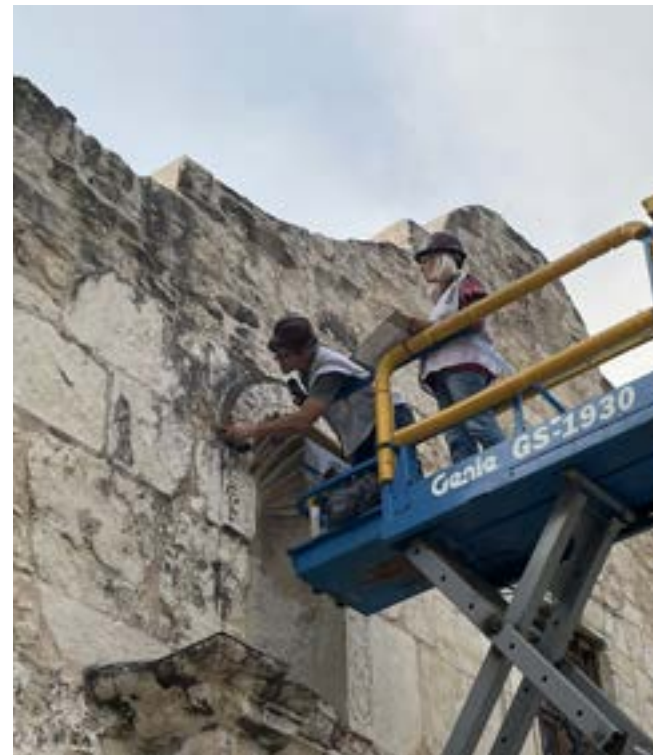
The Alamo conservation team doing work on the front of the Alamo church.
