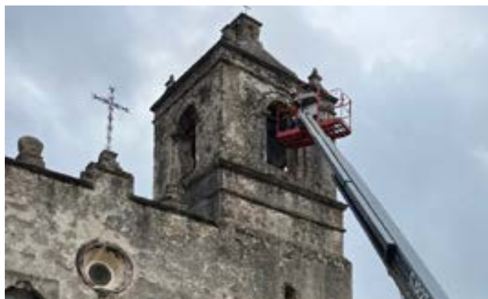
Historic preservation crew works on the bell tower of Mission Concepción's church.
