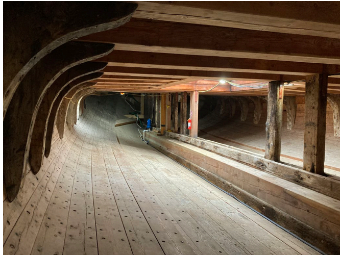
Photo 1. The hold construction is similar to a land-based heavy timber style. This can be difficult to ignite and when ignition does occur, the fire will initially burn along the surface to form a char layer that helps to insulate the timbers from further fire damage. The borate treatment that the Park applies for wood preservation will also function as an intumescent treatment to retard the initial rate of fire spread. The Thayer's hold does not contain a sizable amount of combustible contents that could produce a fast growing fire. The present fire risk is extremely low.
