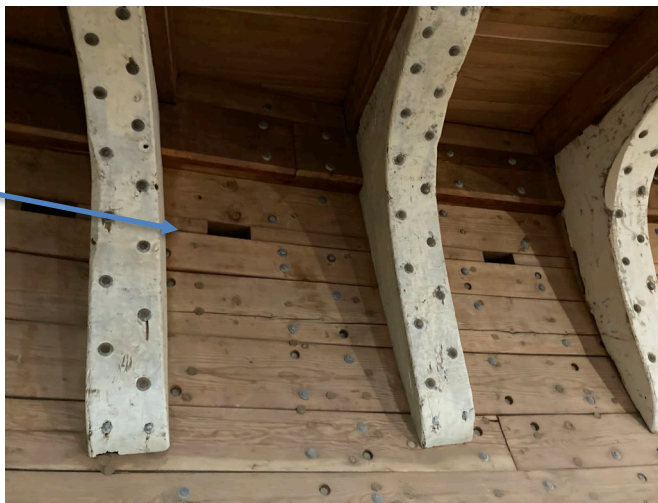
Photo 7: The sampling tubes (0.25 inch/8 mm) can be routed between the futtocks and placed in the shadows of the air vents.
