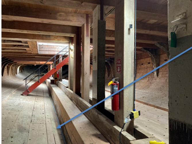
Photo 6: The air sampling smoke detection main tube can be routed under the floor adjacent to the keelson, and the individual sampling tubes run under the floor to the air vents.
