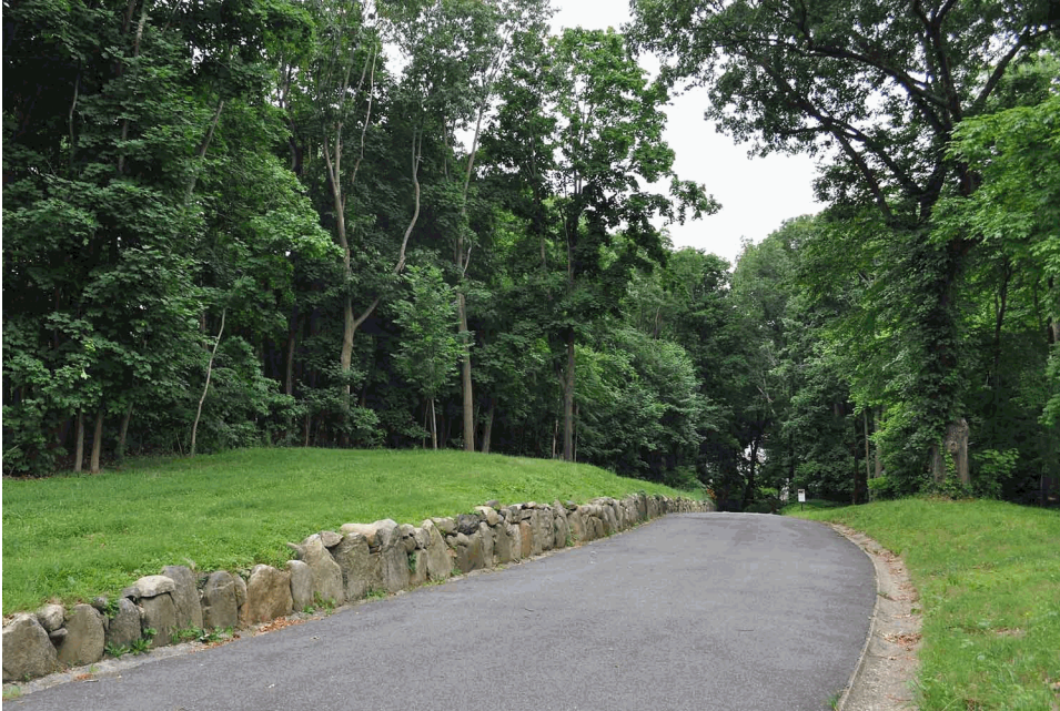
Figure 21. View looking southwest at the Macadam Road and its gutters and stone retaining wall (OCLP, 2013).
