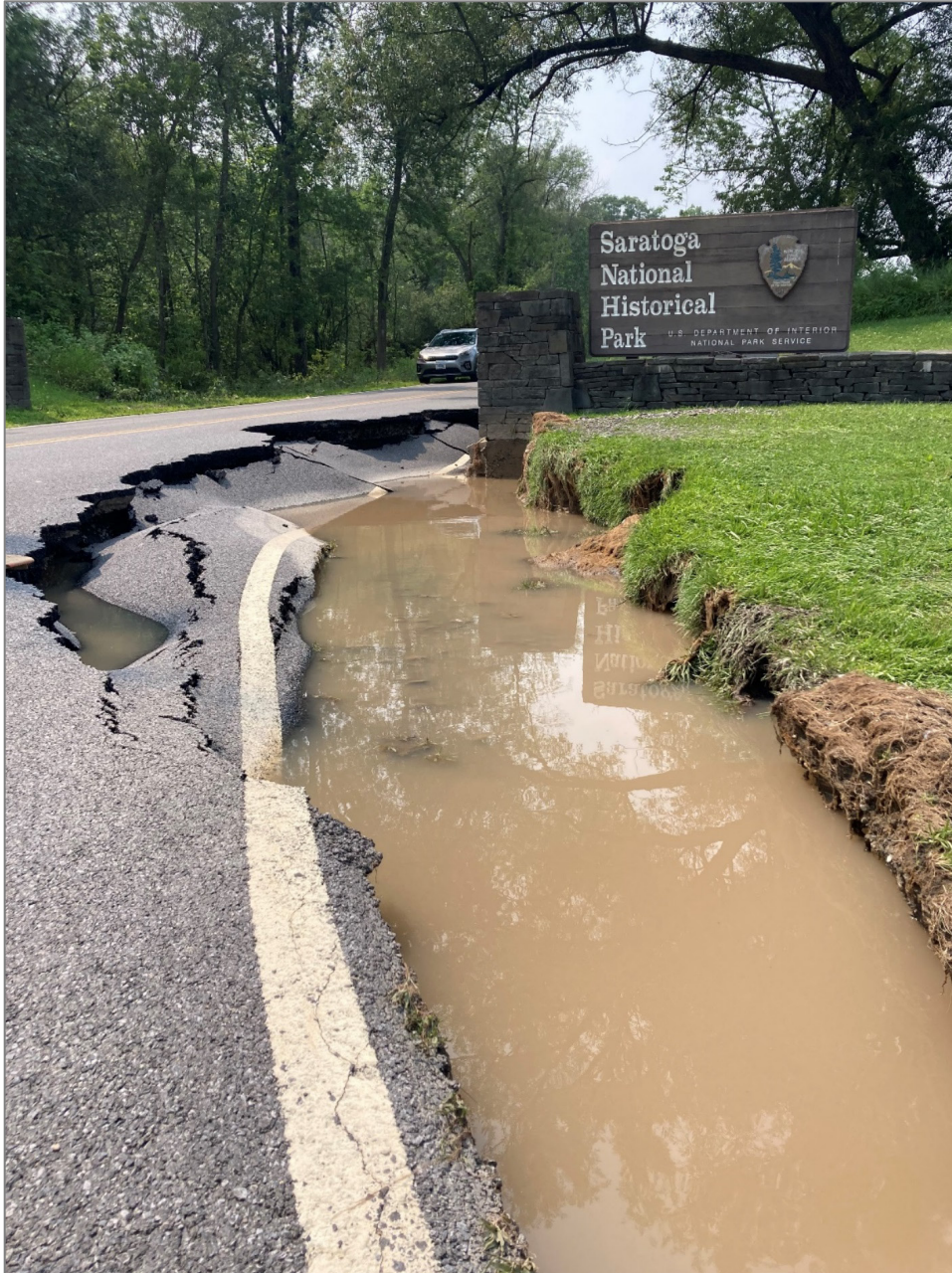
Figure 23. Flash flooding damage along the US Route 4 park entrance. Torrential rainfall that occurred 16 July 2023 resulted in substantial flood damage that washed out portions of the roadway and closed the entrance road and hiking trails. NPS photograph.
