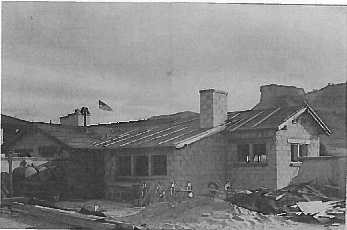
Figure 31. Addition to the Ranger's Residence, under construction, October 16, 1949. Image courtesy of Scotts Bluff National Monument.
