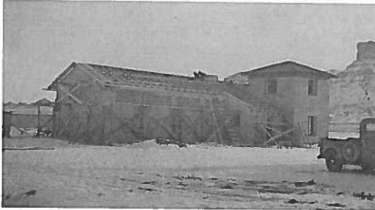
Figure 25. Construction of Paleontology wing and tower addition to Visitors Center, c. 1939. Image courtesy of Scotts Bluff National Monument.
