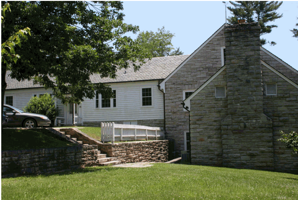
Figure 20. View of stone retaining wall and steps at the west side of the Administration Building (OCLP, 2008).
