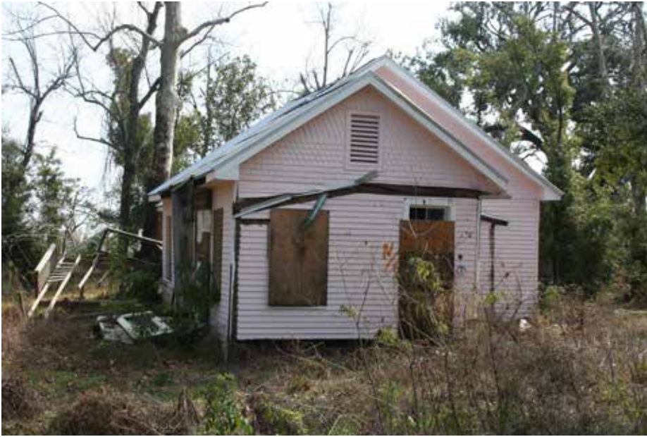
Figure 3: Hurricane Katrina destroyed the wrap-around front porch and knocked the house off the pier foundation. This photo was taken after the site had been cleared and windows and doors were temporarily boarded. Photo: Mississippi Department of Archives and History, Mississippi Historic Resources Inventory (HRI) Database. http://www.apps.mdah.ms.gov/Public
