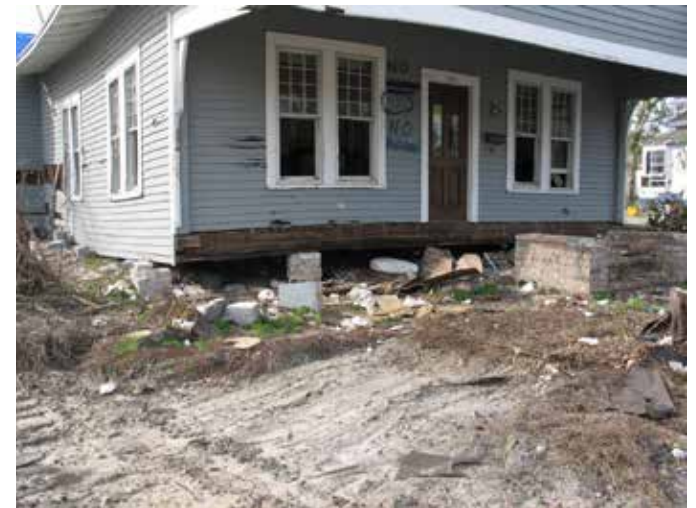
[11] Flood forces are powerful and can result in a building being shifted from its foundation. This historic property in Gulfport, MS, was knocked off of its piers by Hurricane Katrina in 2005. Photo: Jennifer V.O. Baughn/ Mississippi Department of Archives and History, January 26, 2006
