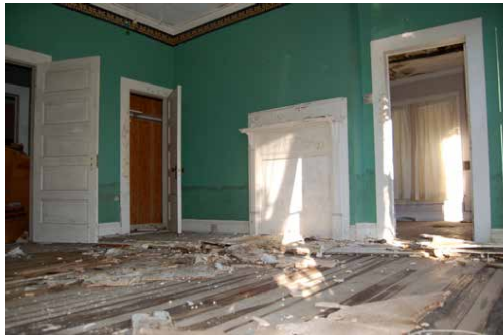
[59] Flood waters can have a significant impact on historic building interiors. Historic features and materials can often be retained and repaired and should not be preemptively removed or replaced. Much of the interior of this flooded historic property in Gulfport, MS, was able to be cleaned and retained.
