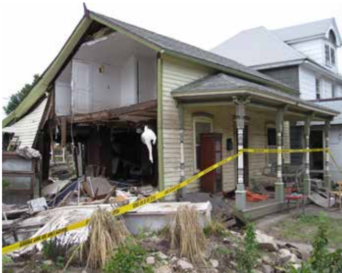
[8] Understanding the characteristics of a flood are critical to understanding property risk. Significant structural damage occurred to this building as a result of a riverine flood in Cedar Rapids, IA, in 2008. Photo: Greg Januska
