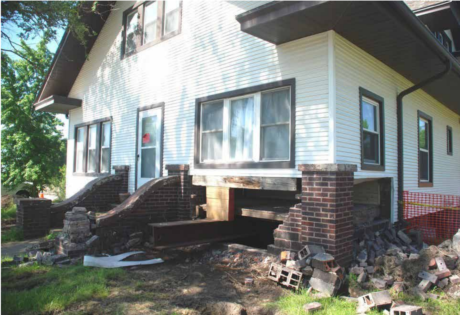
[72] Filling a basement requires access to bring the fill below grade and to maneuver compacting equipment in the space. In this example, a prior flood-damaged section of the foundation wall created an opening that allowed earthmoving equipment access to the basement. The exterior will be repaired once work is complete below grade. Photo: Mitch Paine
