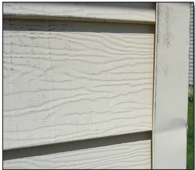
Figure 10—The corner of this house in Soda Springs, ID (Caribou-Targhee National Forest, Intermountain Region), is covered in steel siding that has been battered and bent over the years.
