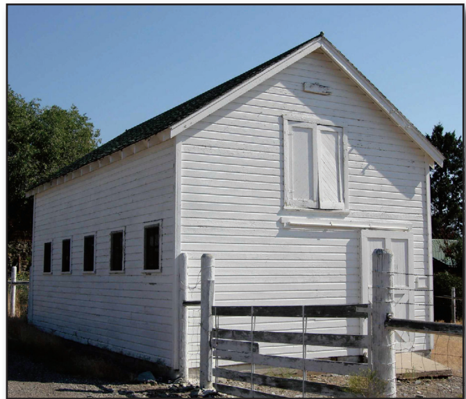
Figure 1—Following national trends, the Forest Service often used wood siding with a variety of profiles on frame buildings in the early 20th century. The drop siding on this barn was one of the most popular choices. The barn was built in 1933 at the Salmon Ranger Station in Salmon, ID (Salmon-Challis National Forest, Intermountain Region).
