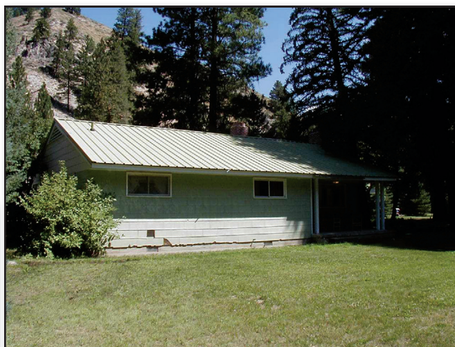
Figure 9—The broken piece of siding shown in figure 8 is from this 1957 house at the Shake Creek Guard Station on the Sawtooth National Forest, ID (Intermountain Region).
