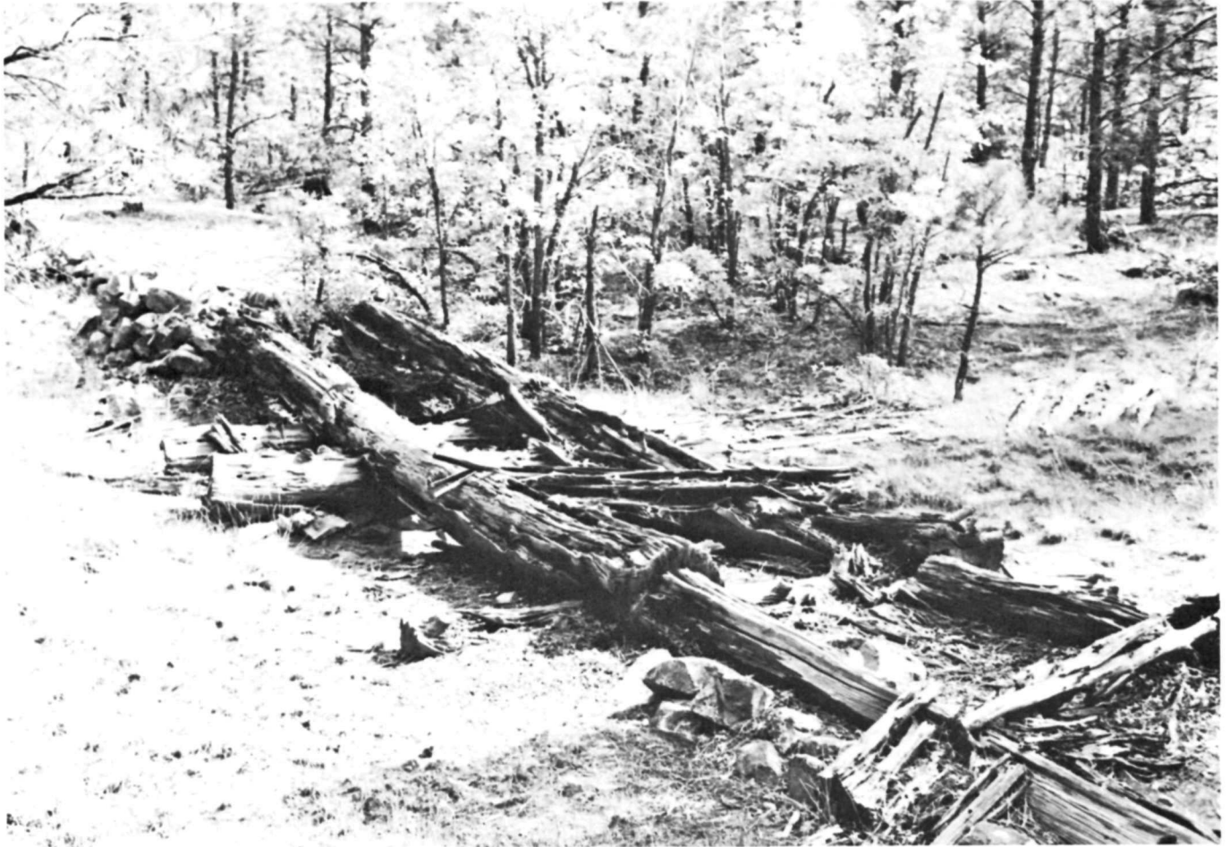
Figure 34. Three span cribwork trestle, 47.9 feet in length, on Pine Canyon railroad of George E. Breece Lumber Company, September 30, 1985. By David "A" Gillio. USDA-Forest Service photograph.
