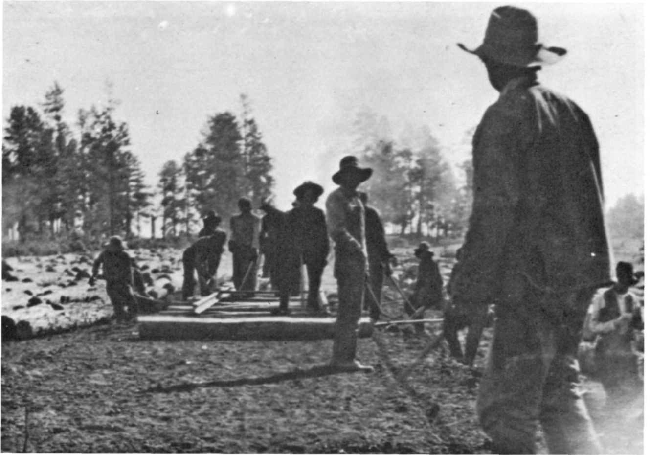
Figure 59. Laying track for the Zuni Mountain Railway on freshly graded roadbed. Logs had already been yarded to both sides of the new spur track ready for loading on the cars. Cibola National Forest collection.
