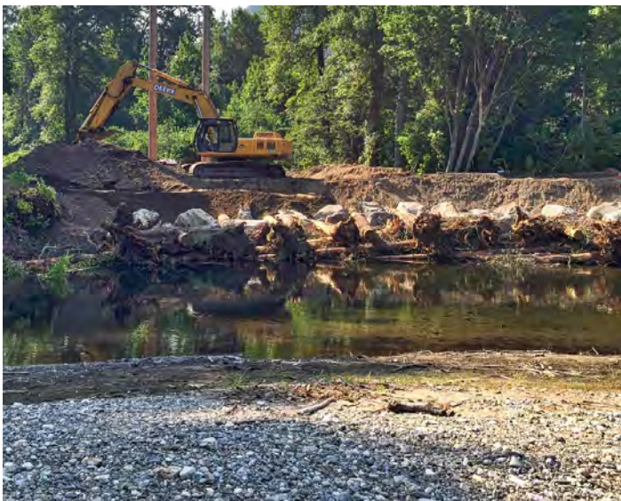
Photo: Meander/ Transmission bend Large Wood Material (LWM). The large wood jam consists of approximately 100 pieces of wood built into an interlocked matrix. The structure was partially excavated into the riverbank along the channel edge with LWM extending into the water.
