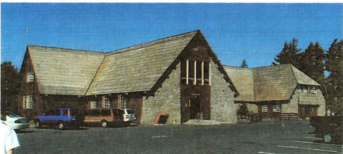
Dave Neville shakes on the roof of the Gift Shop building at the rim of Crater Lake in Crater Lake National Park, Oregon. Photo from: Xanterra Parks & Resorts/Crater Lake
