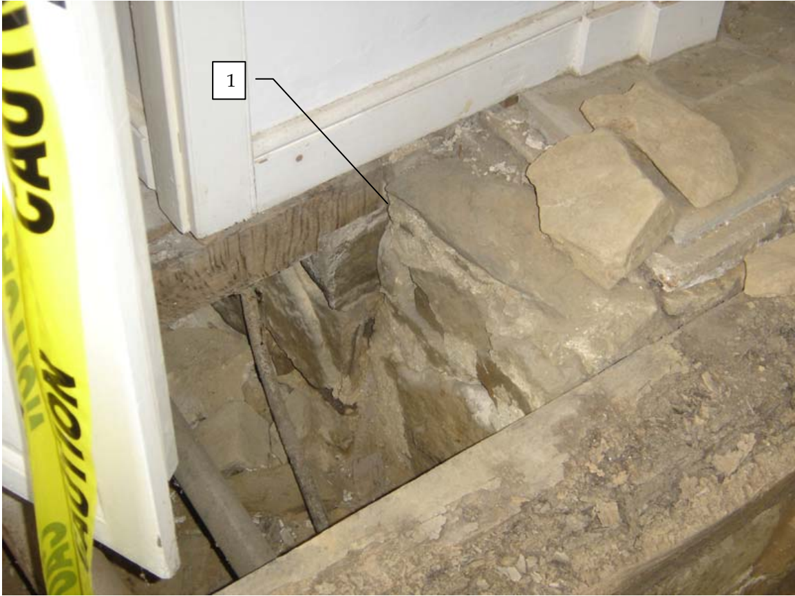
Photo 104d – Detail view of south end of hearth foundation, Room 104, looking northwest.
