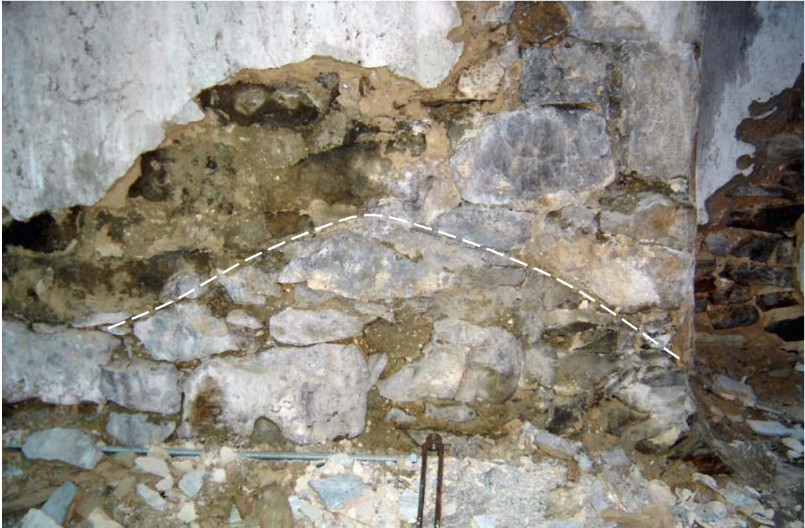
Photo 303b - Chimney mass at west wall, Room 303, looking west. Outline indicates masonry peak corresponding to the peaked ledge at the exterior west elevation of the building.
