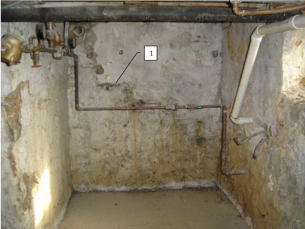
Photo 001a - View of segment of east wall to the south of the chimney vault, Room 001, looking east.
