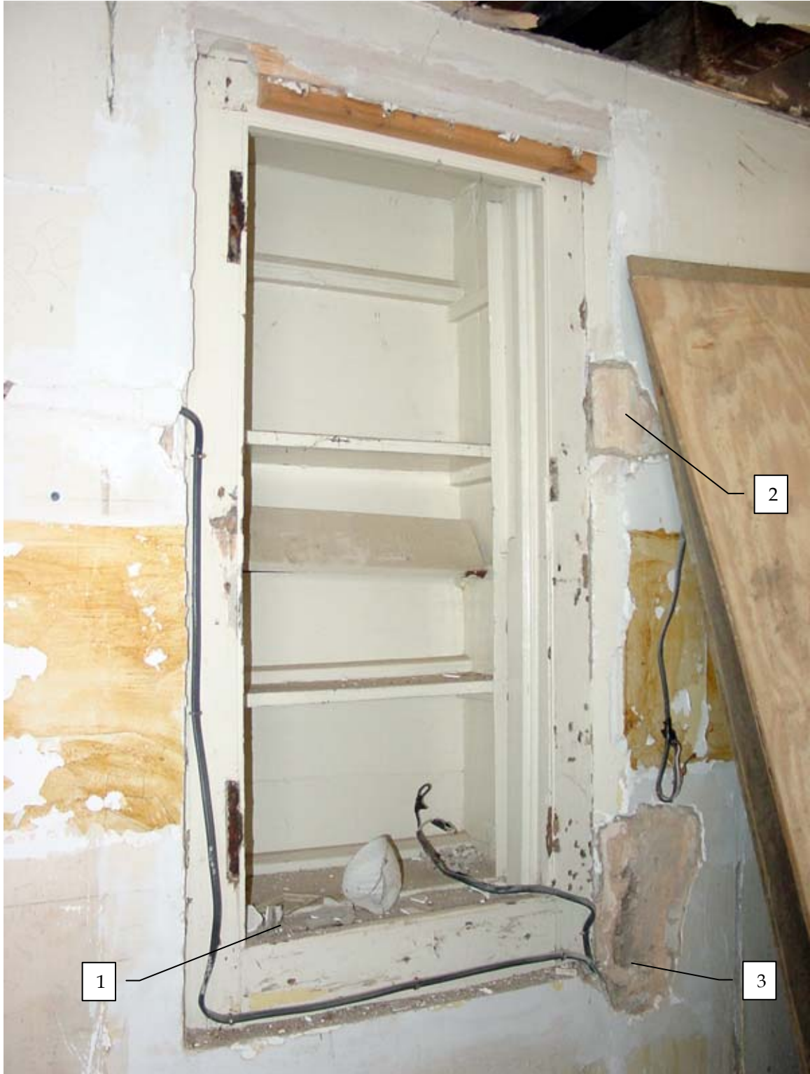
Photo 106b - Built-in cabinet set in original window frame at south wall of Room 106, looking southwest.
