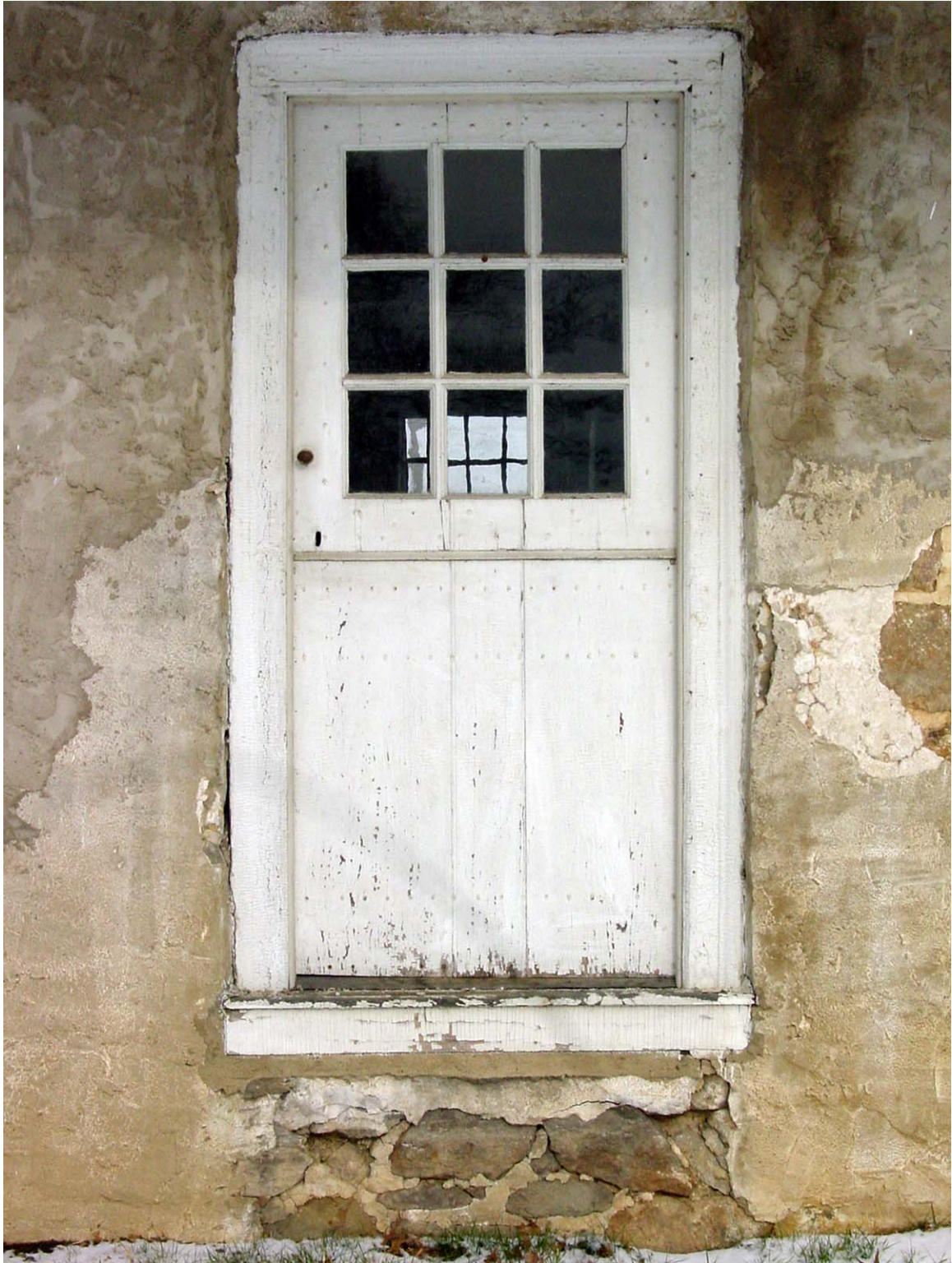
Photo SEc - Exterior view of door to west block, looking north. Wood frame appears to be original. Dutch door is a 20 th century replacement.
