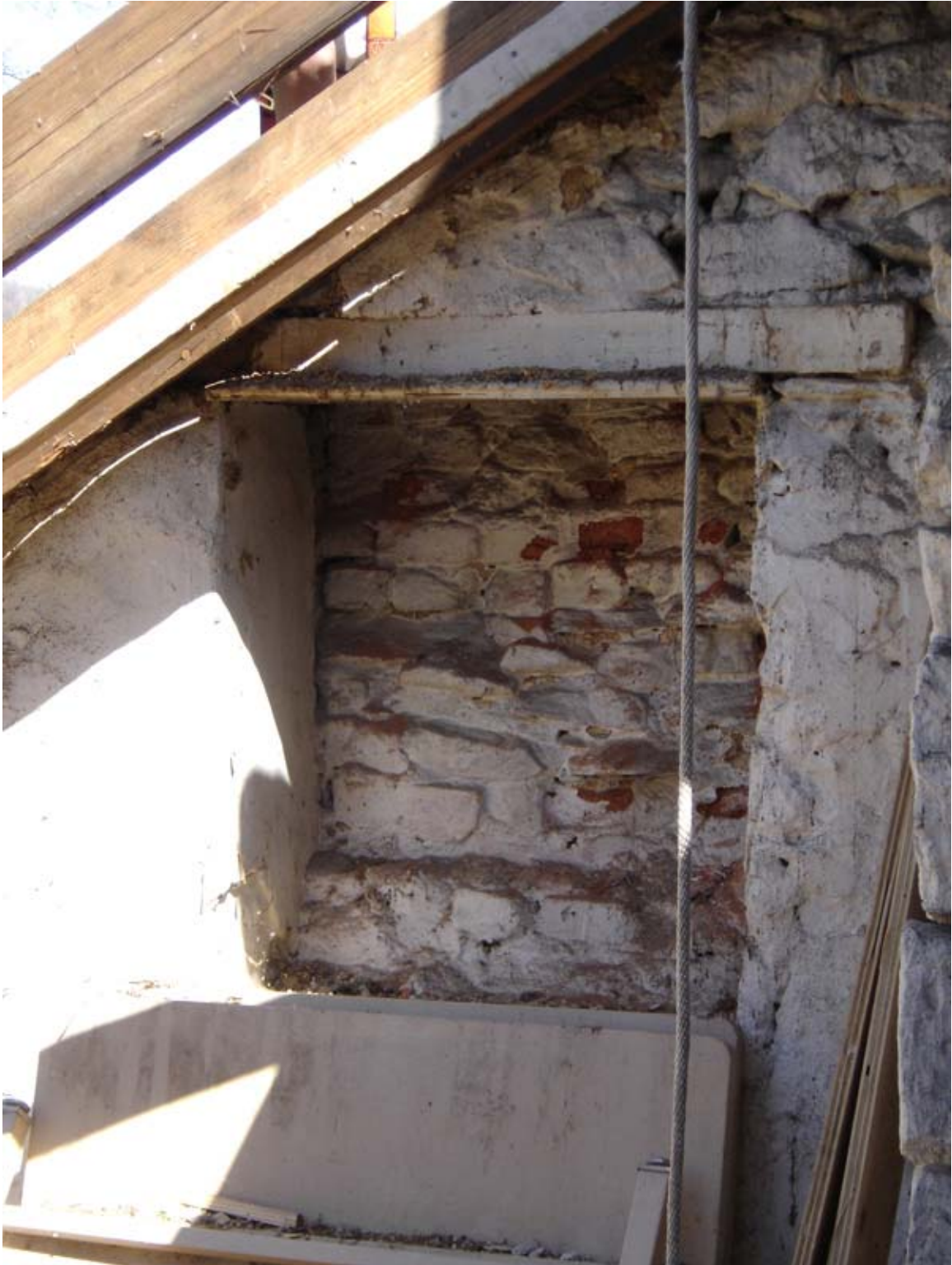
Photo 302b - Interior view of former window opening at east wall, north side of chimney, Room 302, looking east. Opening was in-filled c. 1830 during construction of the east addition.
