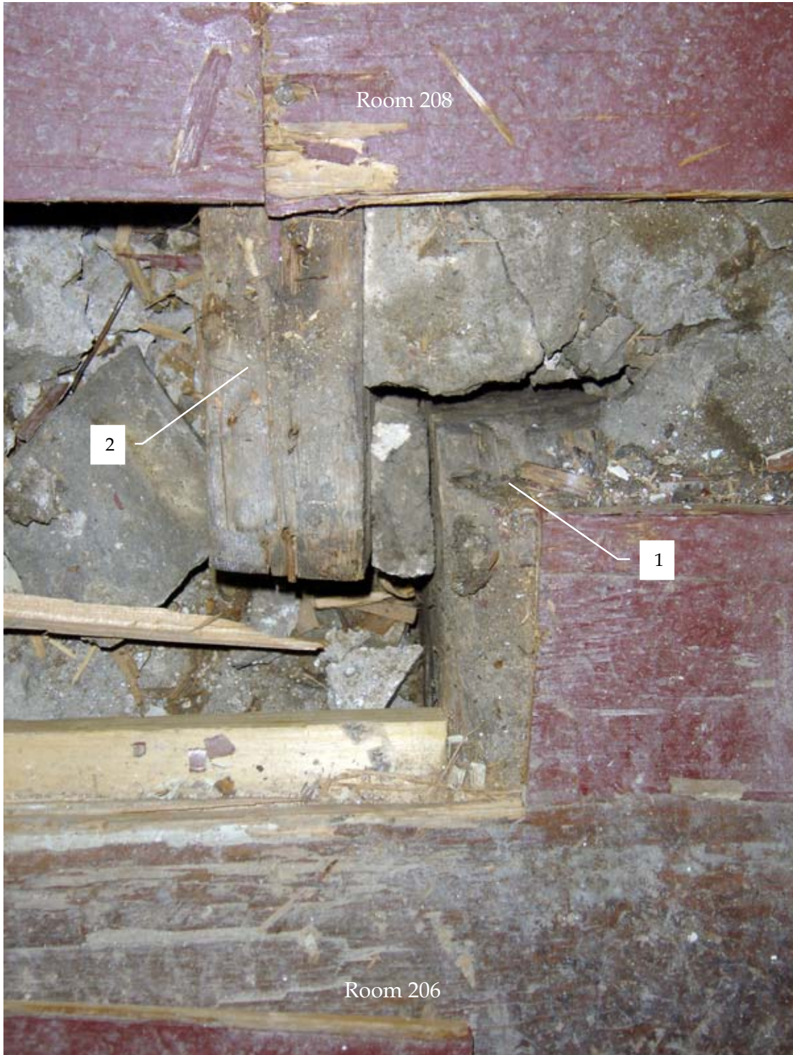
Photo 206d – Detail view of floor and framing (over masonry wall), between Room 206 (bottom) & Room 208 (top), looking down.
