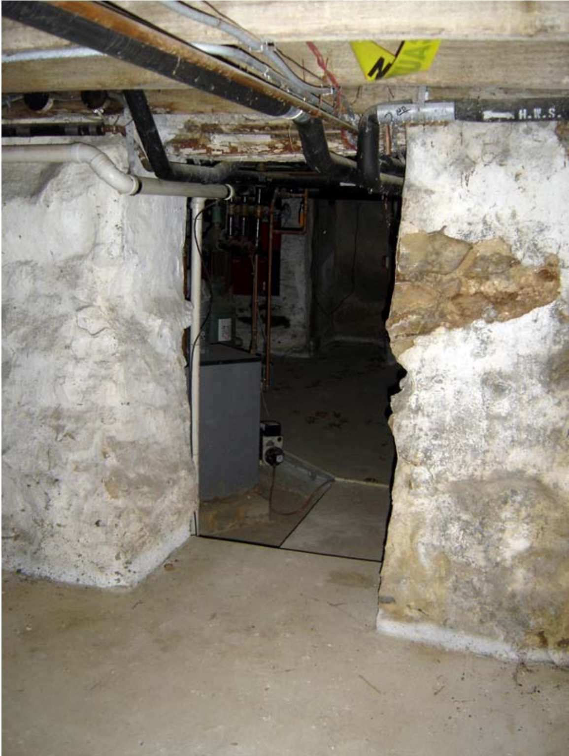
Photo 001b - Masonry opening between Rooms 001 and 002, looking west. Rough character of stonework suggests that the opening was added after original construction. This opening was likely formed at the time of the east addition, c.1830.
