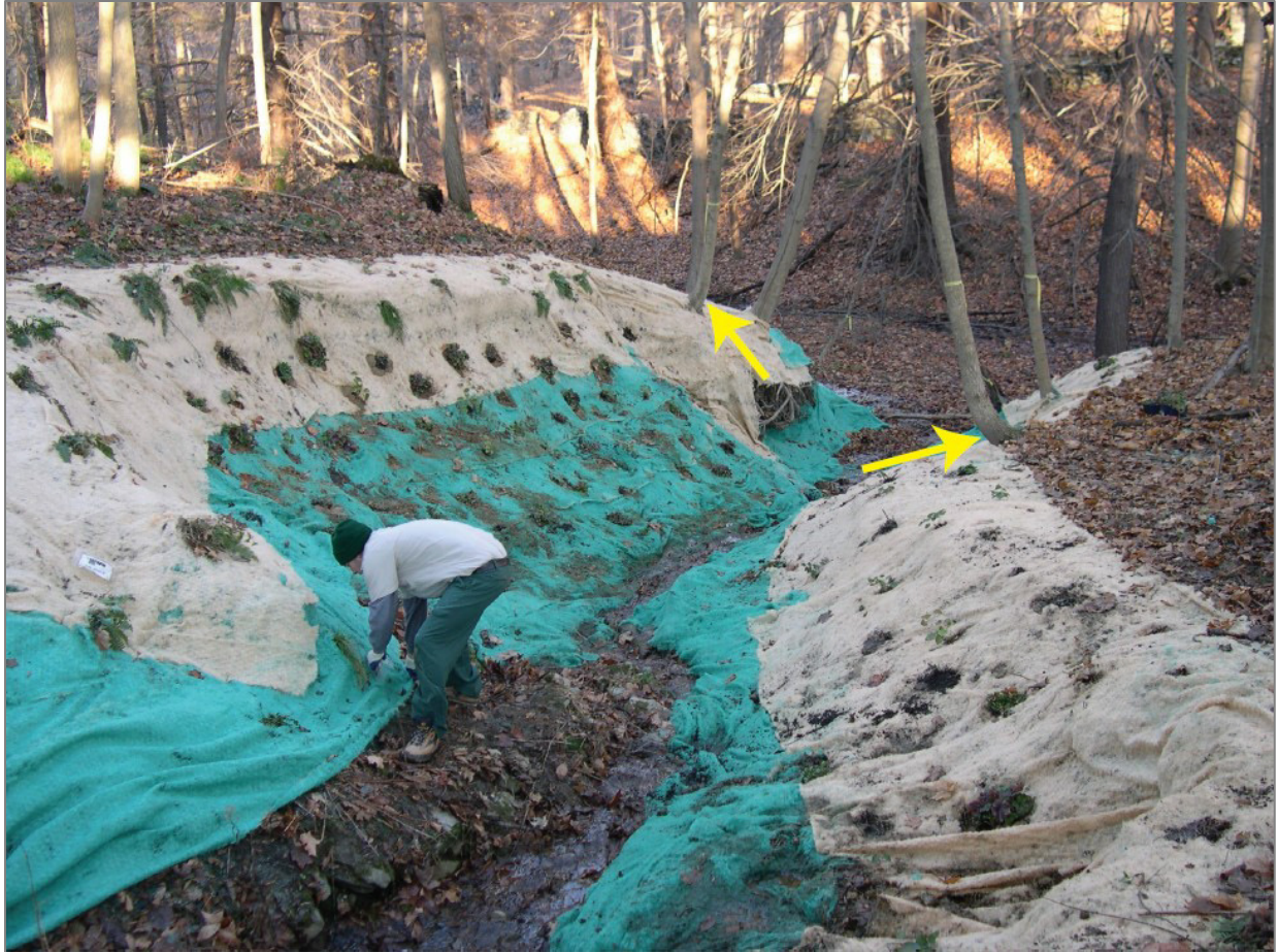
Figure 19. Slope rehabilitation efforts at Home of Franklin D. Roosevelt. Storm drainage adjacent to the FDR Library and Museum has created an erosional swale through part of a historic tree plantation. The 2005 project installed a new catch basin and attempted to stabilize the swale slopes within the damaged site. Indicators of slope instability include leaning and J-shaped trees, such as the ones to the right of the photograph (yellow arrows). NPS / DAVID HAYES
