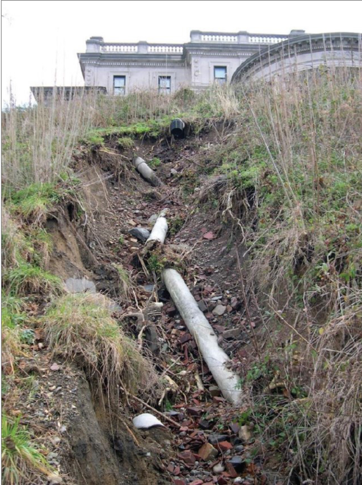
Figure 18. Erosional gully feature created by drainage pipe failure adjacent to the Vanderbilt mansion. Drainage projects engineered to divert precipitation and runoff down the steep slopes next to the Hudson River have caused multiple incidents of erosion and mass wasting. For scale, the drainage pipe at the bottom of the gully is approximately 30 cm (1 ft) in diameter. NPS / DAVID HAYES
