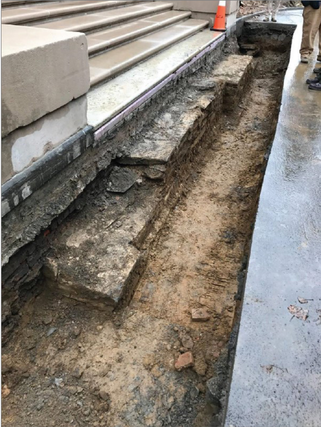
Figure 14. A 2017 archeological excavation in front of the Vanderbilt mansion. The investigation discovered historic foundational structures and artifacts adjacent to the eastern steps of the building. These archeological resources date back to the late 18 th and early 19 th century families that constructed mansions in the same location as the Vanderbilt family. Some of the foundation stones and materials are scorched black from an 1845 fire that destroyed one of the historic mansion structures. NPS / VANDERBILT MANSION NATIONAL HISTORIC SITE
