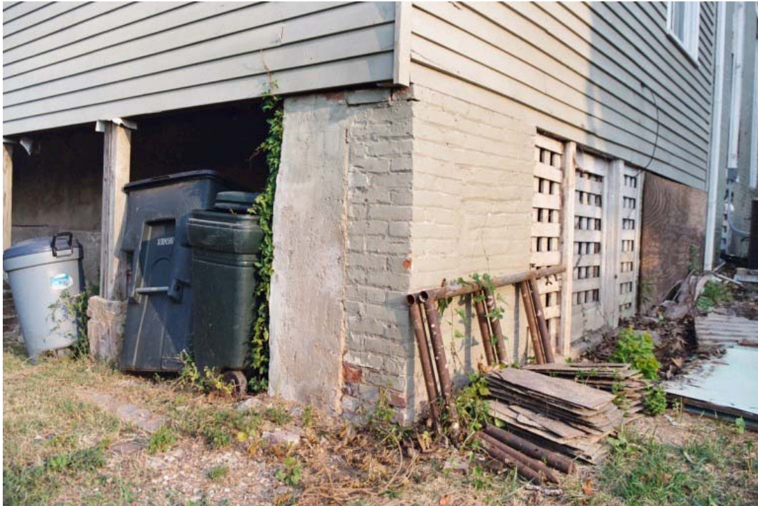
Figure 1 South ell showing added supports for cantilevered floor
