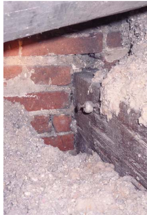
Figure B - 3 Ceiling joists above the original L-shaped porch are resting in formed joist pockets in the brick wall, indicating they are an original feature
