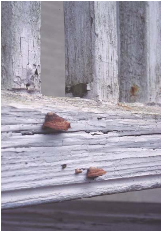
Figure C – 52 Fungus growing on the west porch balustrade
