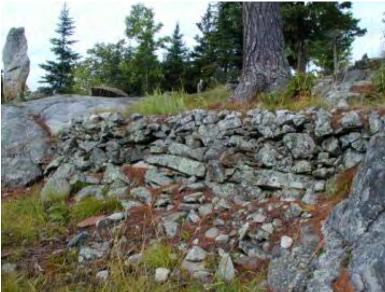
Collapsing stone wall.
