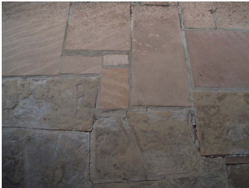
Figure 129. Transition between CCC era and new flagstone on the back porch of the Visitor Center, 2006 (NPS photo).
