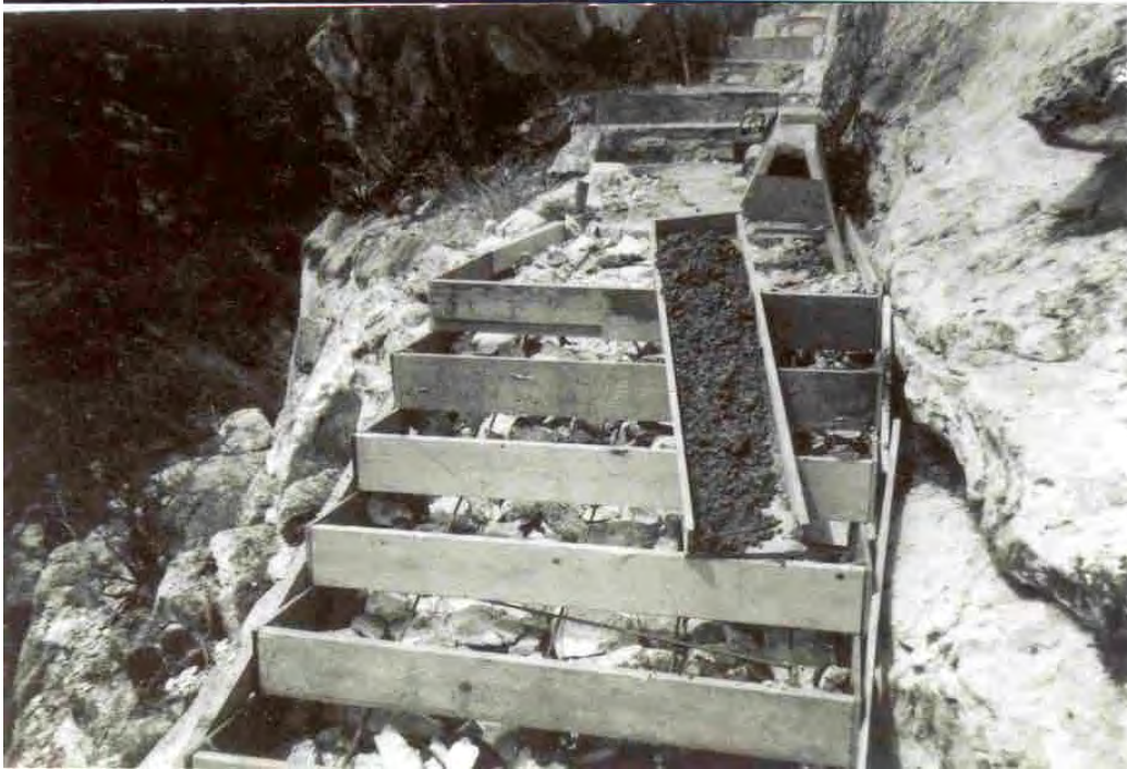
Figure 73. Form for Mission 66 poured concrete stairs, May 1966, note rubble and rebar under form (NPS photo).
