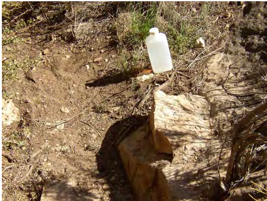
Figure 49. Cement and boulder step in front of WACA 154, along Ranger Ledge trail, 2002 (NPS photo).
