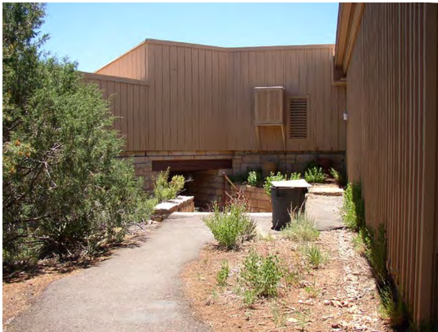
Figure 119. Entrance to the CCC portion of the visitor center with Mission 66 addition (wall on right) and pitched roof, 2004 (NPS photo).
