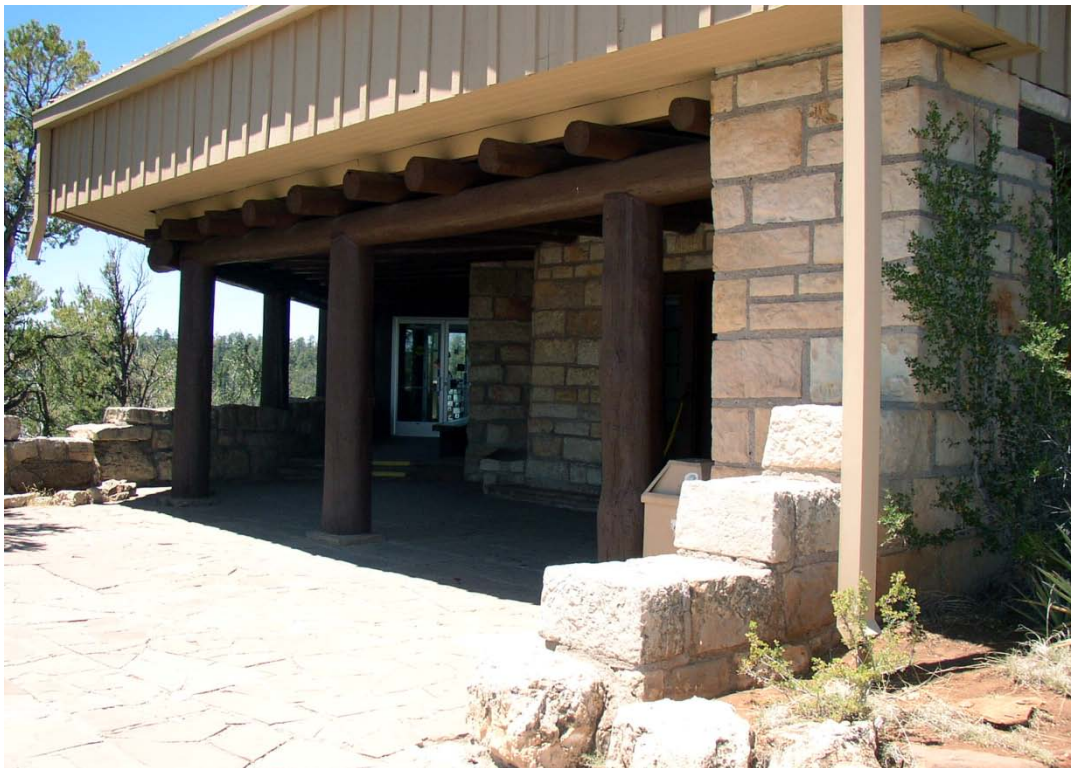
Figure 117. Back Porch of Administration Building with pitched roof, 2004 (NPS photo). The area constructed with limestone is the CCC portion of the visitor center. Note the round vigas.
