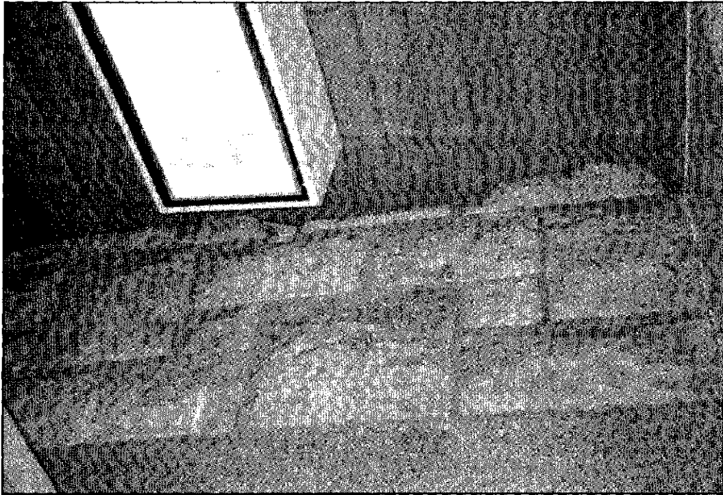
Figure 4.26: Passage, view to northeast with tongue-in-groove wood ceiling scribed to stone building wall.
