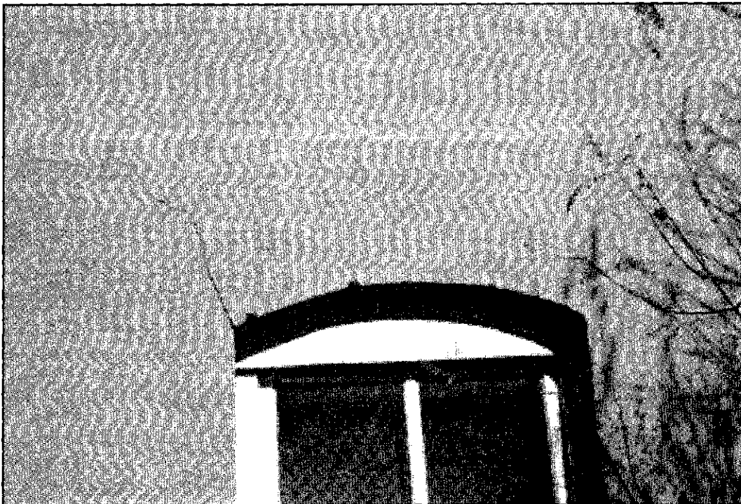
Figure 5.7: Detail of southwest elevation with severe stucco cracking and spots of ferrous staining at window head.
