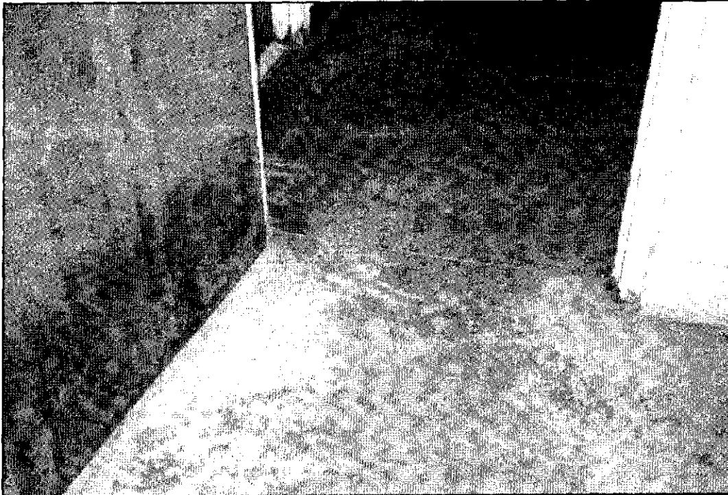
Figure 5.21: Detail of painted concrete floor at door of staff locker room. A large crack beginning at the door frame runs across the opening to an adjacent wall, and the paint has eroded in high-traffic areas.
