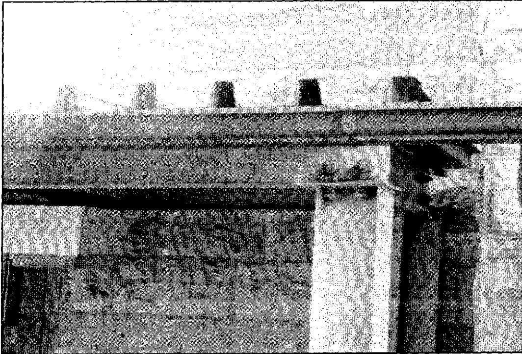
Figure 5.8: Detail of steel structure at northwest areaway roof with failing paint and rust bloom. The K-type hanging gutter and downspout are also experiencing paint failure.
