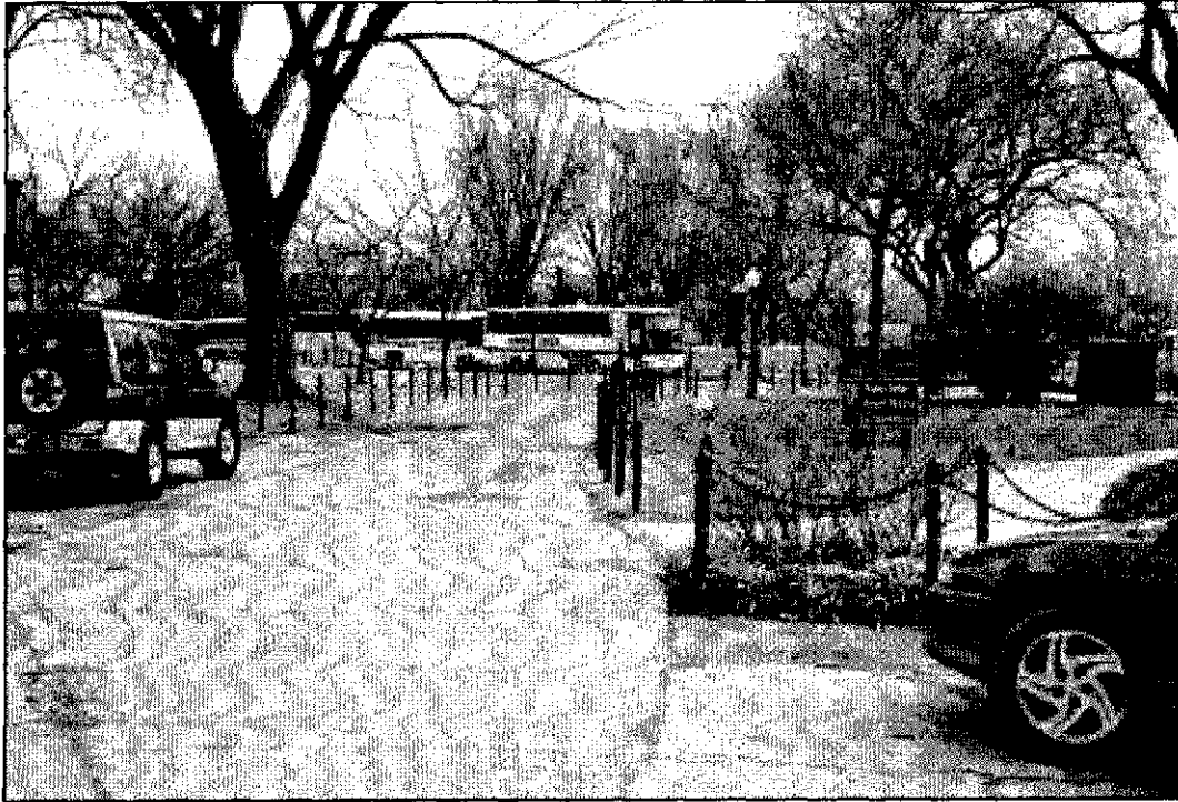
Figure 5.1: Asphalt service drive north of lodge, view to the southeast with serious cracking and previous patches evident.
