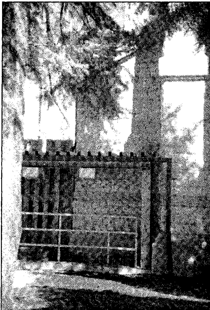
Figure 4.12: Basement areaway roof and handrail with chimney base on right, view to northeast.
