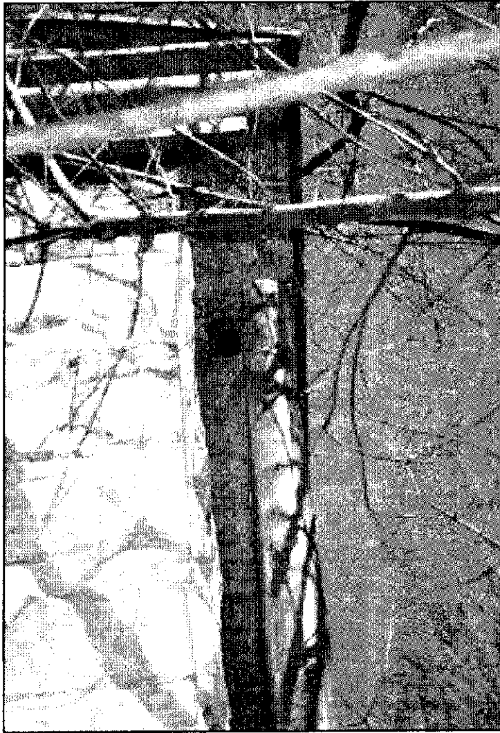
Figure 5.14: Detail of through-cornice downspout disconnected from rain leader at south end of southeast elevation. The downspout is clogged with branches and foliage.
