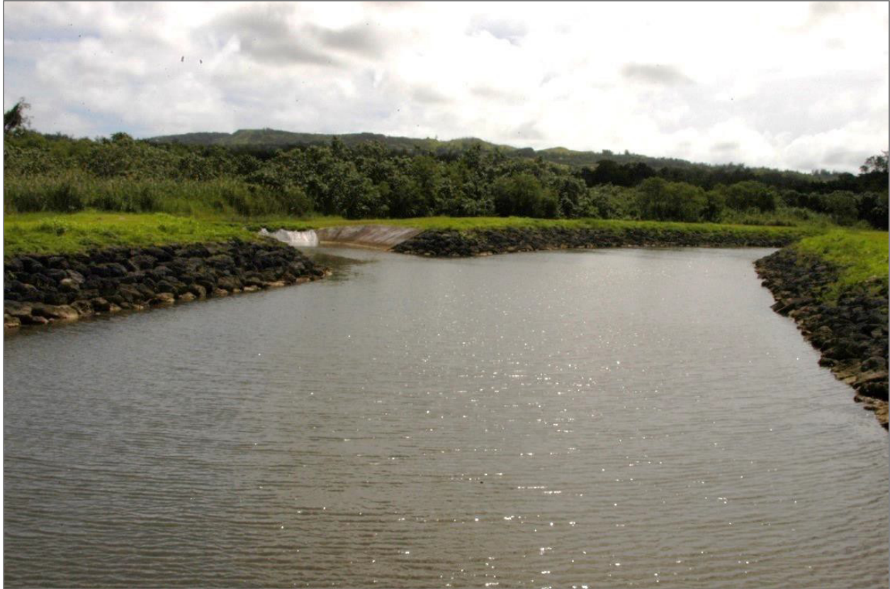
Figure 30. Channelization and streambank enhancement on the Namo River. This reach is adjacent to the Agat Unit, just upstream of the Guam Highway 2 bridge. A spillway that drains a wetland is in the upper left corner of the photograph. (Photo by T.J. Donaldson)
