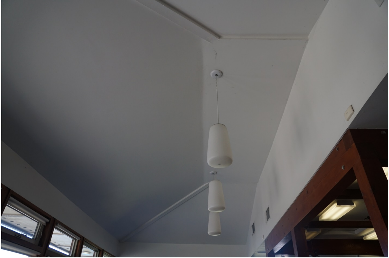
Image 34: Vaulted ceiling in the lobby. Image looking west. Photo by Ashley Phillips.
