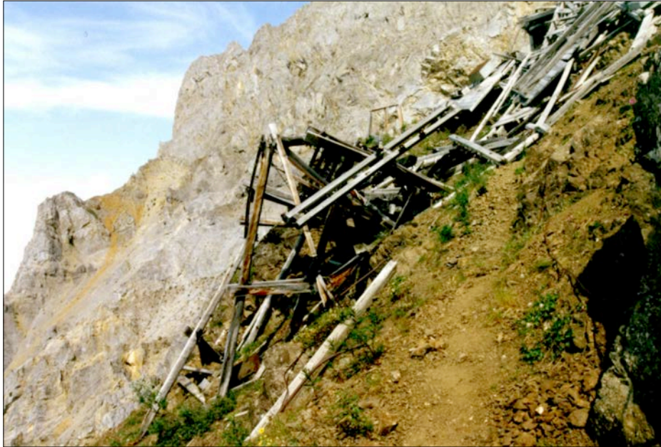
E2: Collapsed tower, view N (NPS, 1993).
