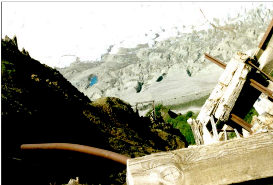
E2: Collapsed tower, view W (NPS, 1993).
