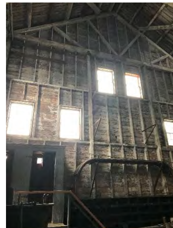
Photo 18 – Power house interior with peeling lead-based paint. Orientation: west. Date: 8/22/2017. Time: 1040.
