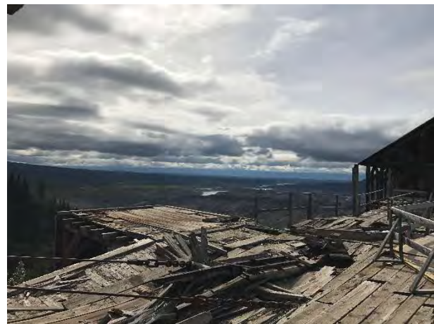
Photo 42 – Collapsing deck of the Mill building, which represents a physical hazard. Orientation: south. Date: 8/22/2017. Time: 1352.
