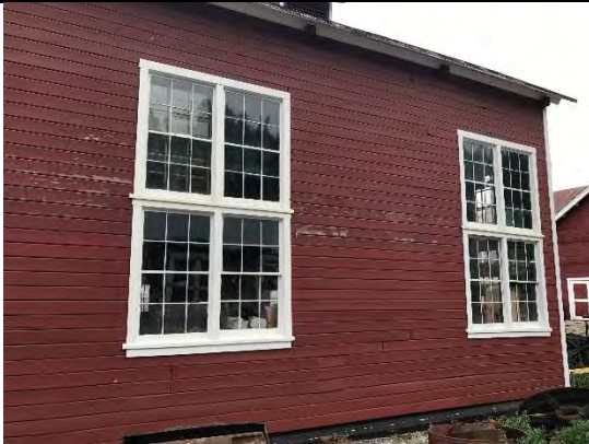
Photo 23 – Peeling lead-based paint on Machine Shop. Orientation: east. Date: 8/22/2017. Time: 1058.
