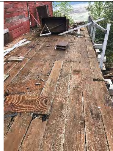
Photo 30 – Western end of the Leach Plant. Note the lack of railing (right) representing a physical hazard. Orientation: west. Date: 8/22/2017. Time: 1007.
