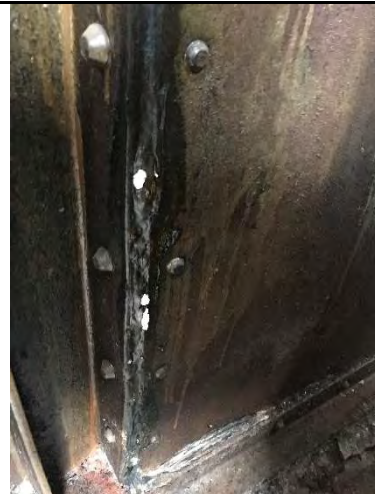
Photo 14 – Cracking of a sealed boiler containing asbestos in the Powerhouse. Orientation: south. Date: 8/22/2017. Time: 1037.
