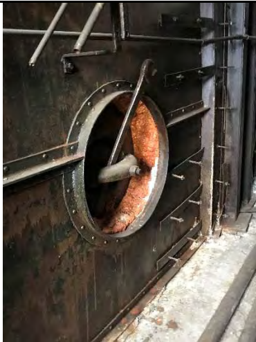
Photo 13 –The seal on a boiler containing asbestos in the Powerhouse. Orientation: south. Date: 8/22/2017. Time: 1036.
