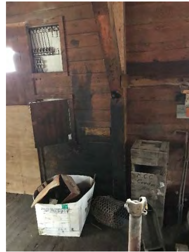
Photo 20 – Asbestos in wall of transformer house. Orientation: north. Date: 8/22/2017. Time: 1050.
