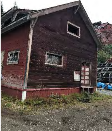
Photo 19 –Exterior of transformer house, painted with lead-based paint. Orientation: northeast. Date: 8/22/2017. Time: 1049.
