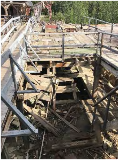
Photo 43 – Collapsing deck of the Mill Building, representing a physical hazard. Orientation: south. Date: 8/22/2017. Time: 1354.
