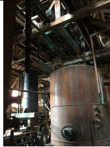
Photo 32 – Ammonia tanks in Leach Plant. Note green staining on ceiling beams. Orientation: northwest. Date: 8/22/2017. Time: 1122.
