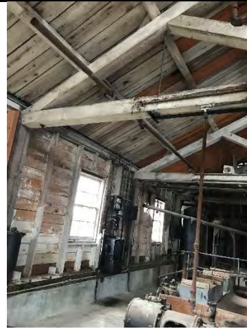
Photo 12 – Power house interior with peeling lead-based paint. Orientation: west. Date: 8/22/2017. Time: 1022.
