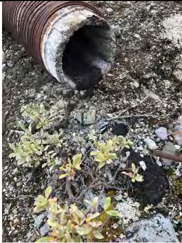
Photo 11 – Sewer line and soil staining. Orientation: east. Date: 8/22/2017. Time: 1018.
