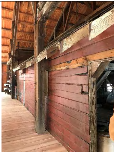
Photo 29 – Leach Plant interior with new ceiling and original lead-based paint. Orientation: southeast. Date: 8/22/2017. Time: 1105.
