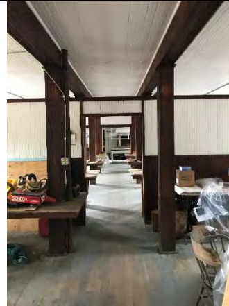
Photo 58 – Peeling white paint on ceiling and grey arsenic-containing paint on floor of the West Bunkhouse. Orientation: southwest. Date: 8/22/2017. Time: 1149.
