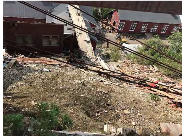
Photo 44 – Debris by the Mill Building. Blasting caps, representing an explosive hazard, have been found in the debris. Orientation: west. Date: 8/22/2017. Time: 1429.
