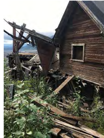
Photo 40 – South side of Mill Building. The debris and collapse potential are physical hazards. Orientation: northwest. Date: 8/22/2017. Time: 1345.
