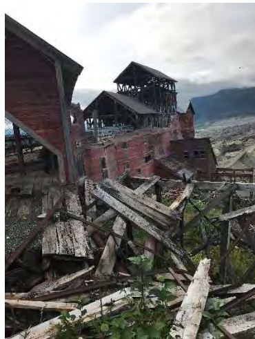
Photo 37 – Tramway building and Mill Building. Field contains debris, and building exterior contains lead-based paint. Orientation: south. Date: 8/22/2017. Time: 1344.
