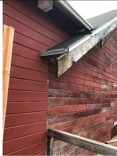
Photo 28 – North end of Leach Plant showing repainted (left) and original lead-based paint (right). Orientation: south. Date: 8/22/2017. Time: 1105.
