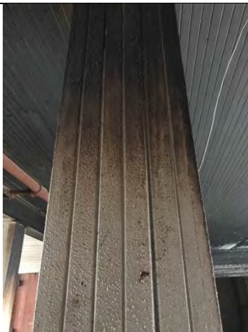
Photo 59 – Basement of the West Bunkhouse. A historic fire caused the white paint to “boil.” Orientation: NA. Date: 8/22/2017. Time: 1200.
