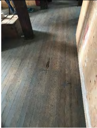
Photo 57 – Gray paint that contains arsenic on the floor of the West Bunkhouse. Orientation: north. Date: 8/22/2017. Time: 1149.
