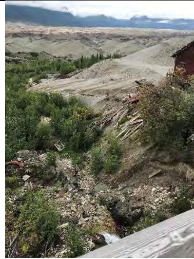
Photo 36 – National Creek (center) and Leach Plant (right). Building debris is actively falling into the creek. Orientation: east. Date: 8/22/2017. Time: 1131.
