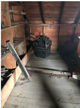
Photo 21 – Lead battery in transformer house. Orientation: north. Date: 8/22/2017. Time: 1052.
