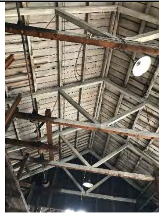
Photo 26 – Peeling lead-based paint on ceiling of Machine Shop. Orientation: NA. Date: 8/22/2017. Time: 1100.
