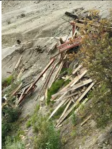
Photo 35 – Slope west of Leach Plant. A seep (left) runs under the Leach Plant creating a collapse potential. Orientation: southeast. Date: 8/22/2017. Time: 1130.
