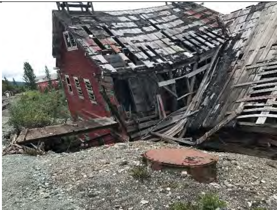
Photo 33 – Exterior of Leach Plant. The collapsing structure is a physical hazard. The wall contains original lead-based paint. Orientation: south. Date: 8/22/2017. Time: 1125.
