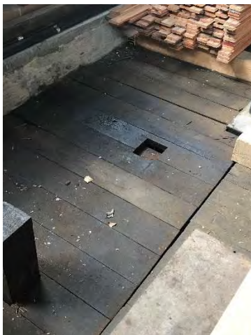
Photo 17 – Bunker C staining underneath the day tank in the powerhouse. Orientation: west. Date: 8/22/2017. Time: 1026.
