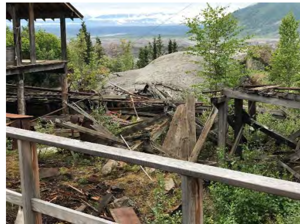
Photo 22 – Debris next to the Machine Shop which represents a physical hazard. Orientation: south. Date: 8/22/2017. Time: 0919.
