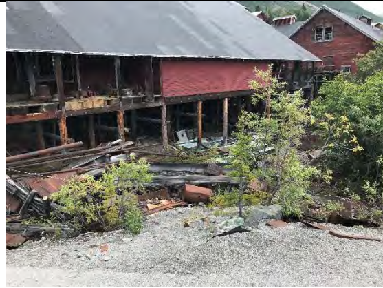
Photo 24 – Boiler Ash cap (foreground), machine shop, and leach plant (right). Orientation: south. Date: 8/22/2017. Time: 1007.
