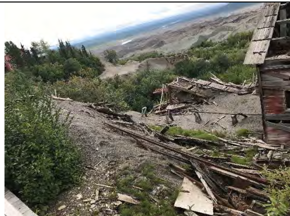
Photo 34 – Debris by west end of Leach Plant (foreground) and unknown surface water feature (background) downgradient of the Mill Site. Orientation: south. Date: 8/22/2017. Time: 11218.
