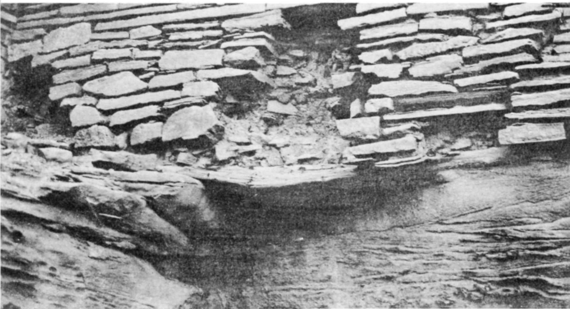
Pole-supported wall before repair, above you at Stake 5.
