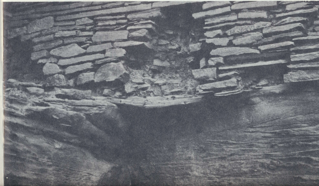
Pole-supported wall before repair, above you at Stake 5.
