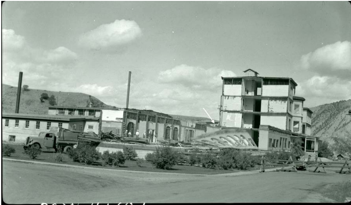
Figure H-5. Looking east towards the old Mammoth Hotel being razed to make way for the new dining room and lounge buildings, take August 14, 1936. The roof of the 1913 wing, the only portion of the old hotel left standing, is indicated by the white arrow. (Photo No. 31109; Box X-29, Freezer 1, Yellowstone Photo Archives.)
