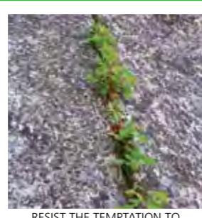
RESIST THE TEMPTATION TO REMOVE PLANT LIFE FROM CRACKS
