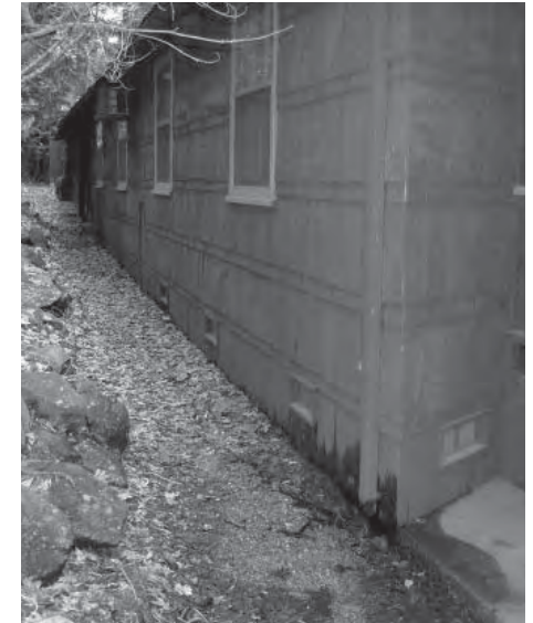
Moisture damaged shakes on rear porch, 2006.
