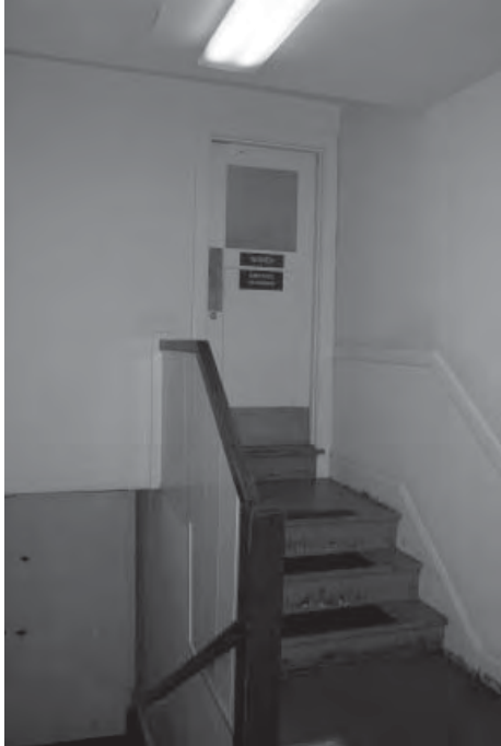
Example of inaccessible bathrooms, 2006.
