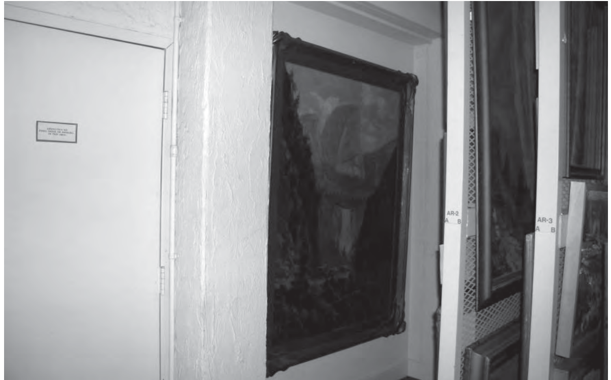
Former doorway from library to lobby (center of photo, new door on left), 2006.
