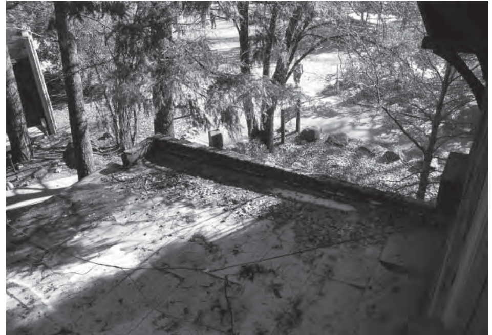
East wing, note accumulation of debris, 2006.
