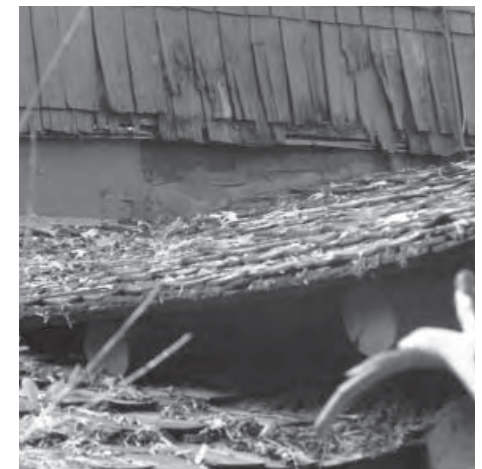
Deterioration above north porch, 2006.
