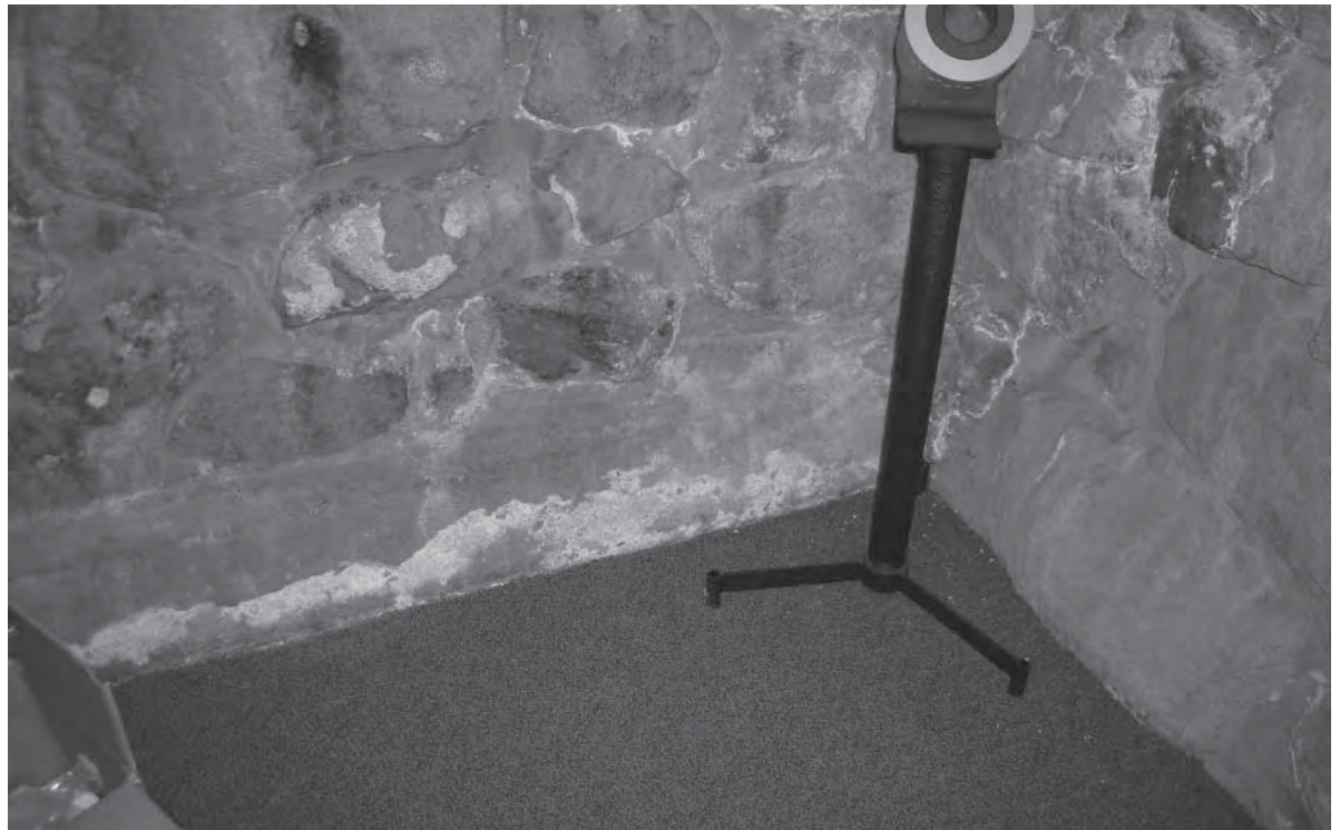
Efflorescence in SE corner of briefing room, 2006.
