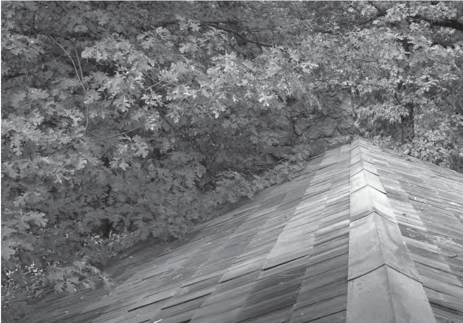
West wing, tree branches in contact with roof, 2006.
